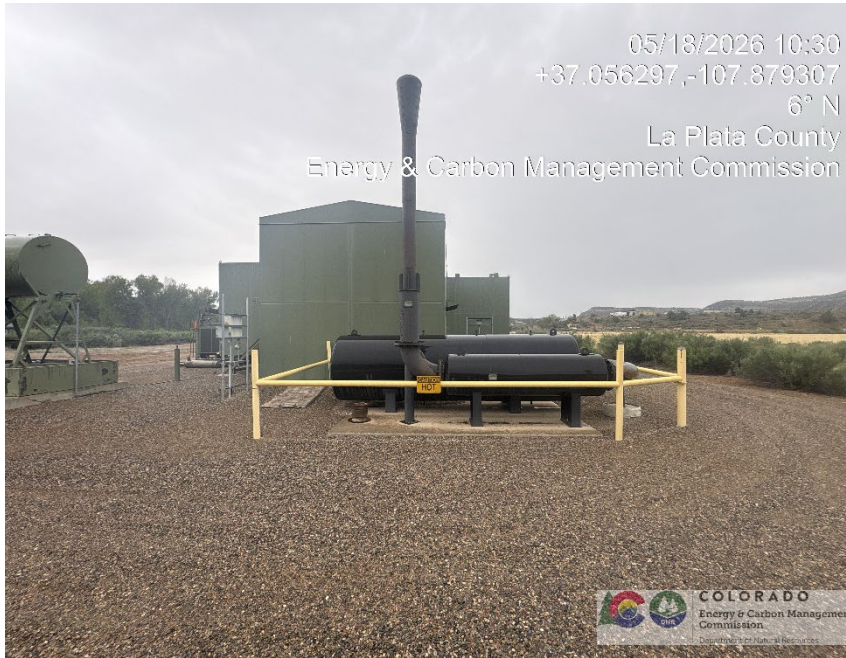
11. Compressor station with 2 stage silencer.
