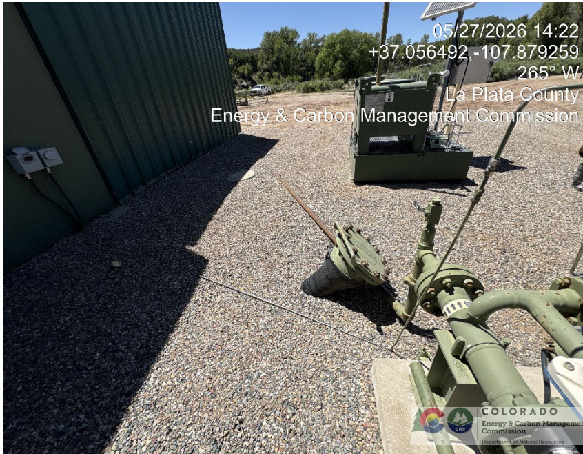
33. Chemical injection tank, 8 inch gas line with 19" blank flange.
