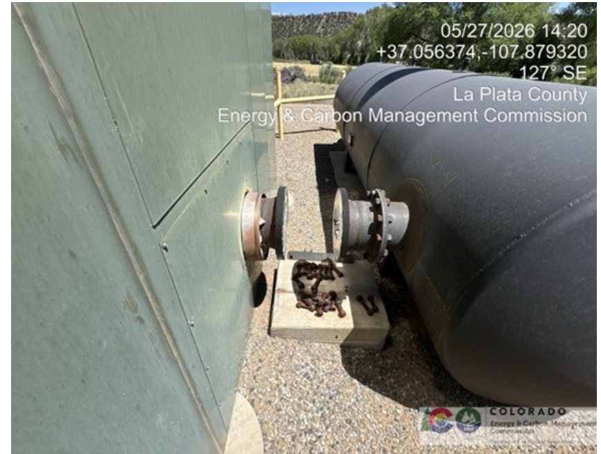
12. Two stage silencer is disconnected.
