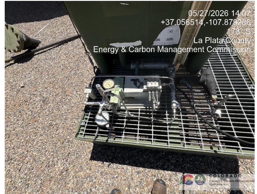
38. Detail of chemical injection container controls. Some stainless tubes disconnected. Unclear if in-use.
