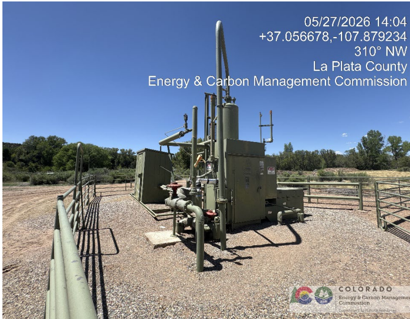
39. Vertical heated separator and associated flow lines. Appears to be anchored in at least 3 locations by turnbuckles attached to concrete pilings buried in the ground.
