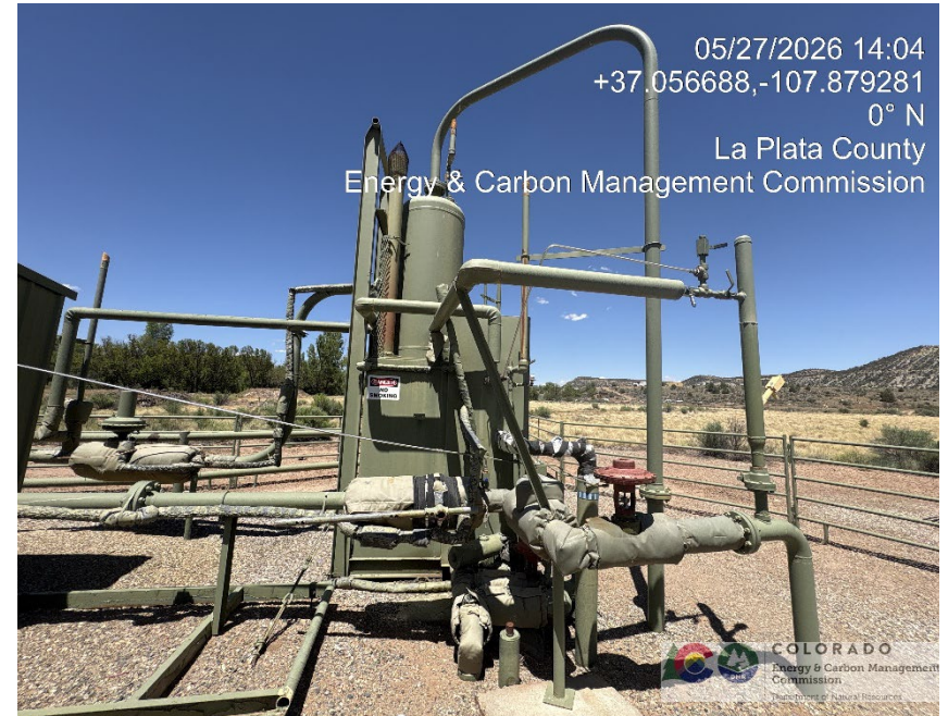
40. Vertical heated separator.
