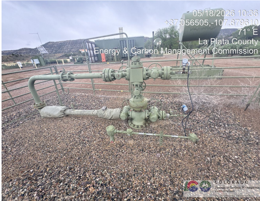
7. Wellhead. Note dead vegetative debris in fence.
