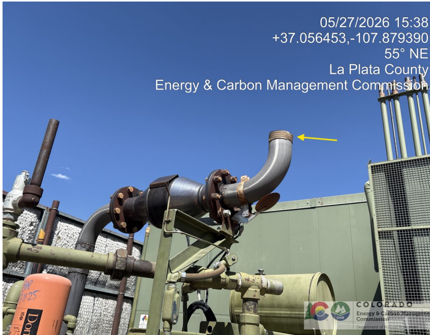
23. Exhaust stack on compressor is missing muffler. Yellow arrow shows flexible exhaust pipe remnants. Loud.
