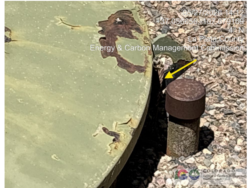
28. Anchor tie down point for 21 BBL PBV tank.
