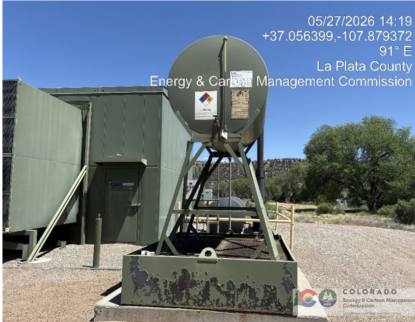
31. Lube oil tank on secondary containment. Is not anchored for potential flooding. There is a ball valve drain at the base connected to an open-ended rubber hose that rests on the ground several yards away. See photo 32
