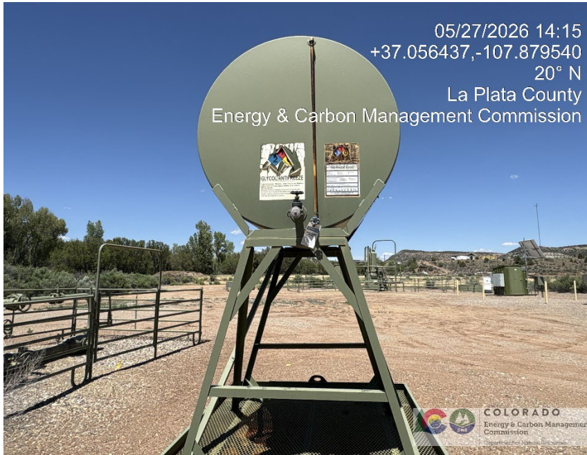
35. Glycol/antifreeze tank with spill prevention. Sight glass cloudy, unknown if contains product. In floodplain. Not anchored. Appears like it may not be in use.
