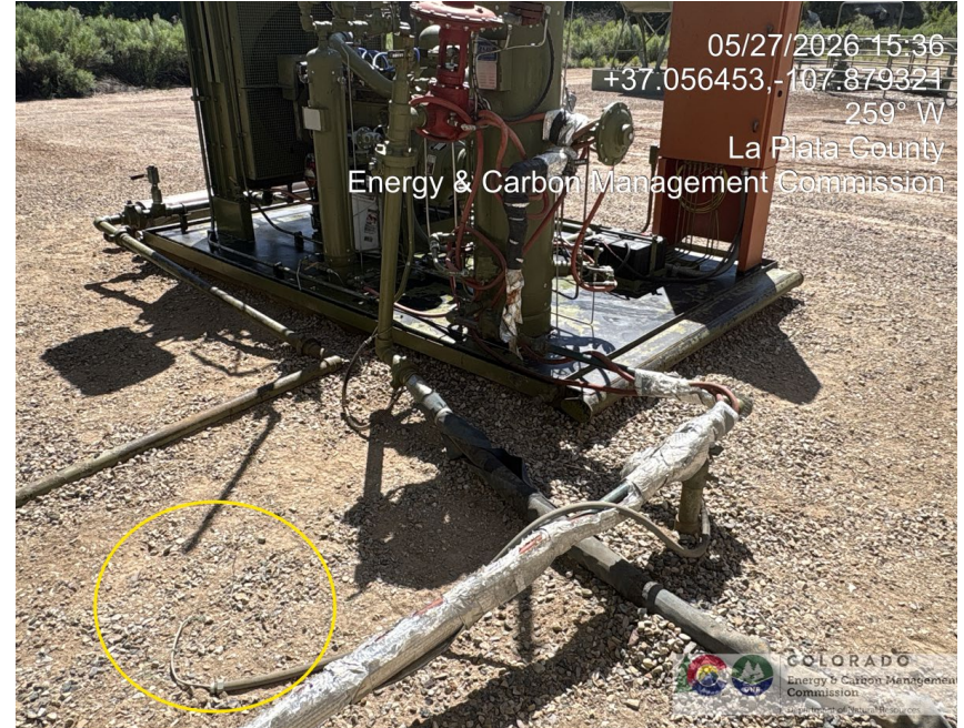
26. Frayed, disconnected wires protruding form conduit near skid mounted compressor.
