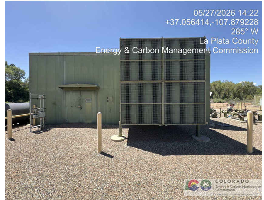
20. View of east side of compressor station looking west. Cooling system on right.
