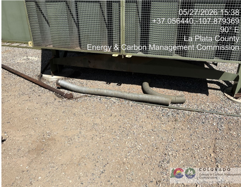
25. Segments of exhaust tubing from compressor. Also shows open ended lube oil hose from lube oil tank
