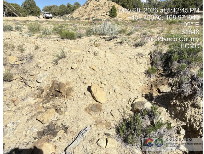
Photo # 5818 Erosion & sediment migration with staining/insufficient BMP's
