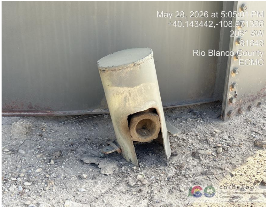
Photo # 5808 Open ended load line
