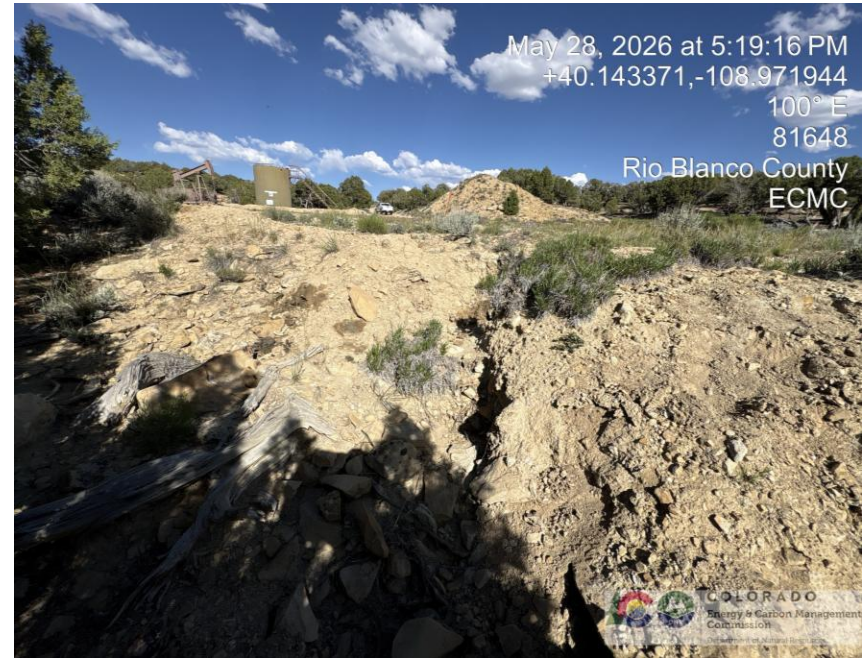
Photo # 5827 Erosion & sediment migration with staining/insufficient BMP's
