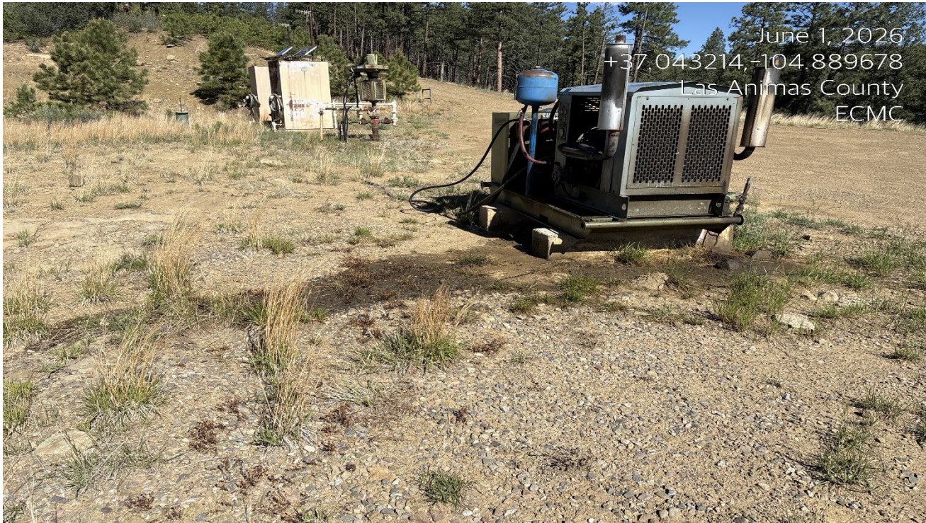
Photo 4. There is oily fluid that spilled on the ground and oily fluid in the engine skid that needs to be cleaned up..
