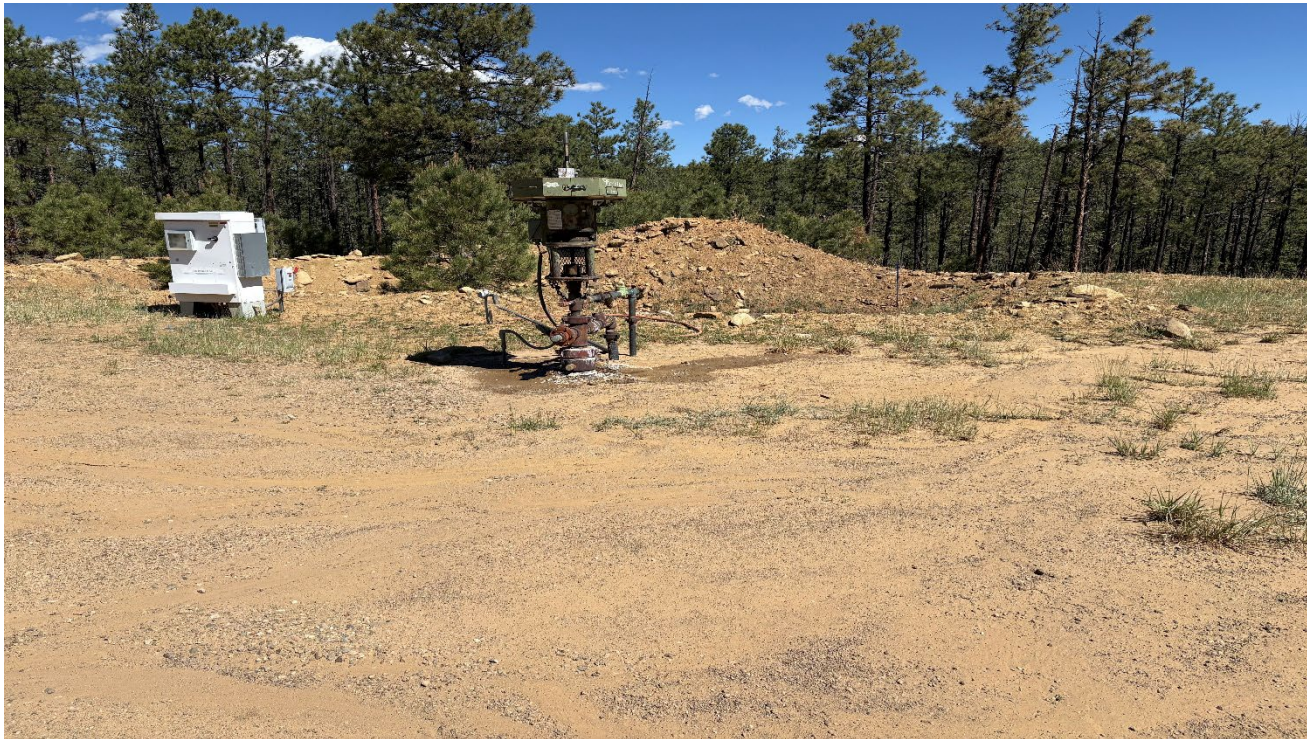
Photo 3. There is a dripping leak at the wellhead that needs to be fixed.
