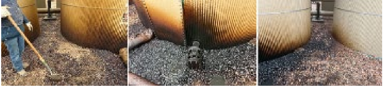
Photo Date 5/28/2026- Spill discovery and start of impact removal
