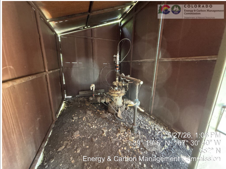
Wellhead inside housing
