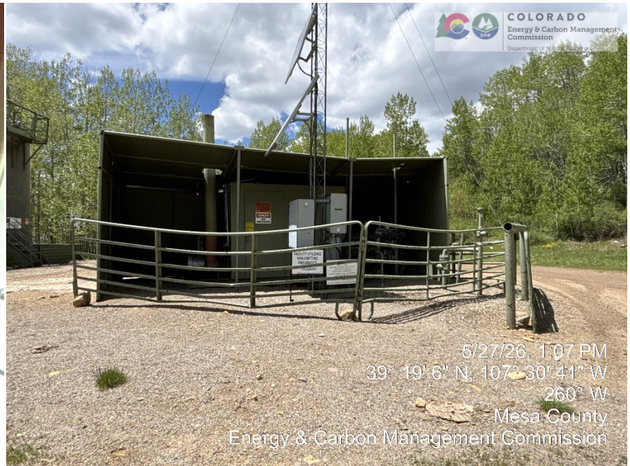
Separator with fence and signs Telemetry
