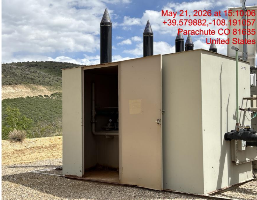
Unsecured Separator/Wildlife Entry Hazard – Photo #03990
