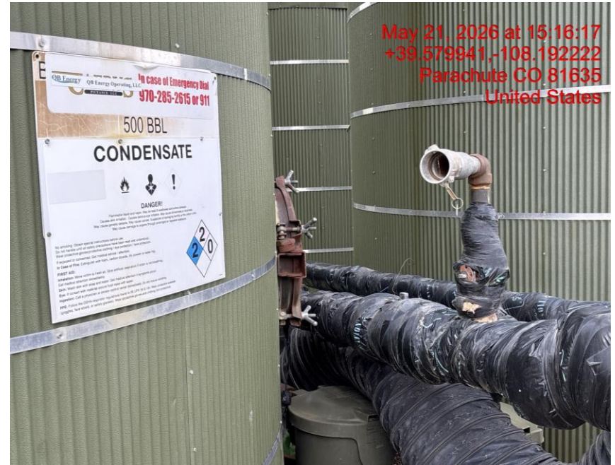
Unplugged Line – Photo #04006
