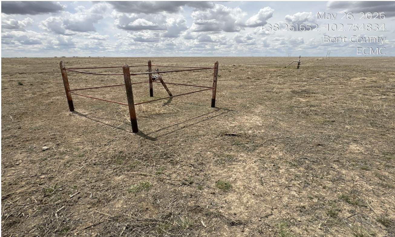
Photo 2. Facing west at the location. The abandoned pipe risers have not been removed.
