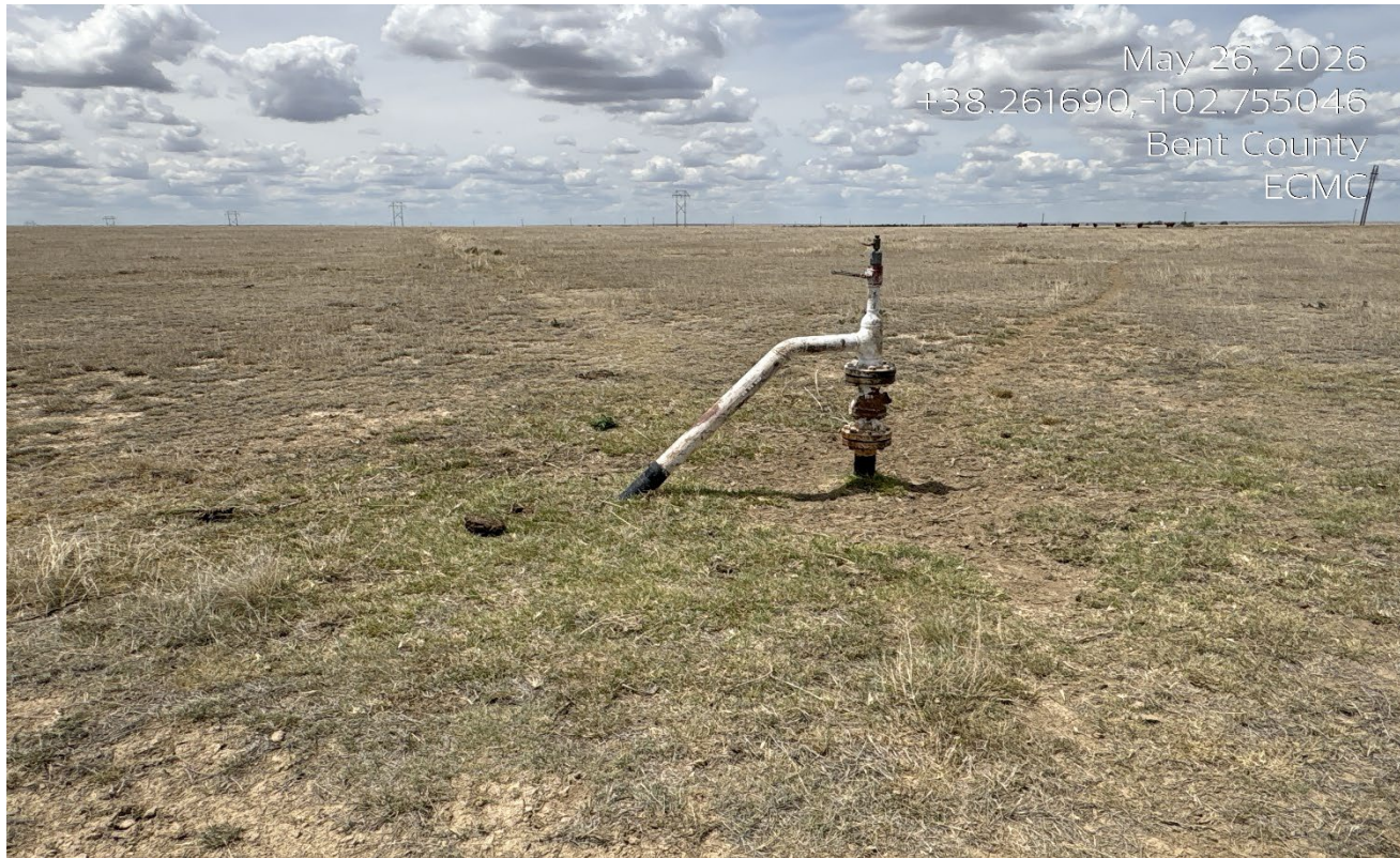
Photo 6. This pipe riser has no signage or LOTO.
