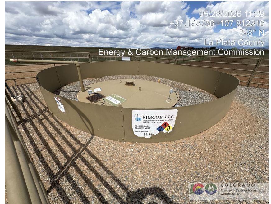
10. Linder A2 95 BBL produced water tank. Tank label is peeling.
