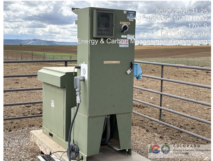
20. Linder A4 electric controls.
