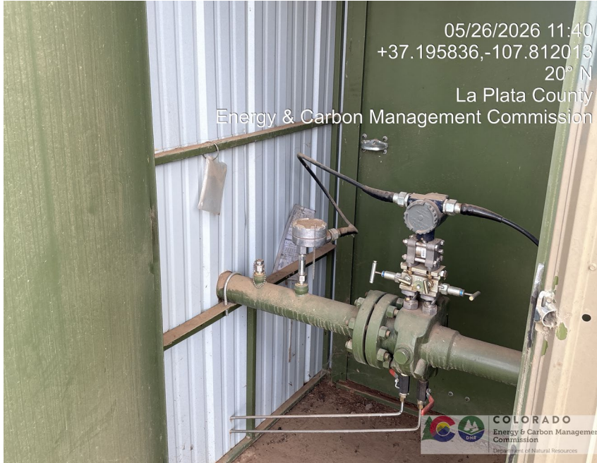
23. Meter run for A4. Both ¼" stainless vent tubes connected to ball valves in this meter shed.
