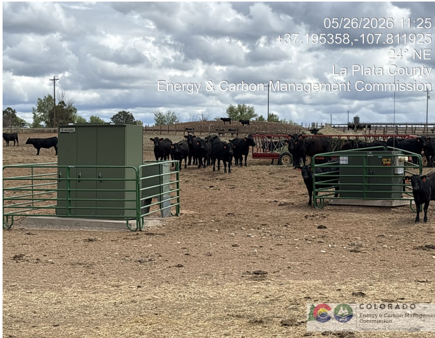
27. Electrical control panel and electric service behind individual cattle panel fence.
