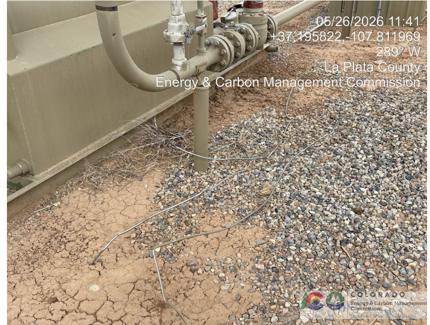
26. Stainless tubing on ground not in use.
