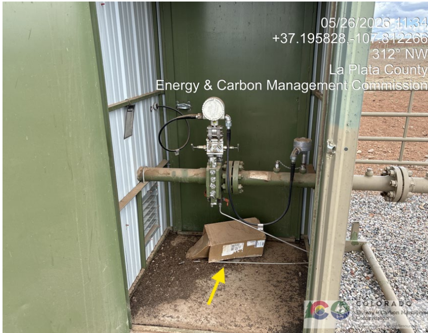
15. Inside A2 meter run shed. On 1/4" vent line is disconnected (yellow arrow). Gas could vent inside enclosure. Cardboard trash on floor.
