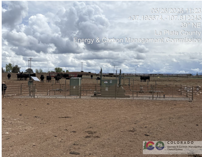
21. Linder A4 production equipment. L-R: Solar telemetry, meter run, horizontal heated separator and flow line.
