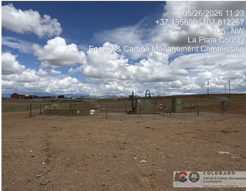
9. Linder A2 production equipment behind cattle panel fence. From left to right: 95 BBL produced water/natural gas PBV tank, horizontal heated separator, meter run, and solar telemetry. Various flow lines, mostly 3" diameter.
