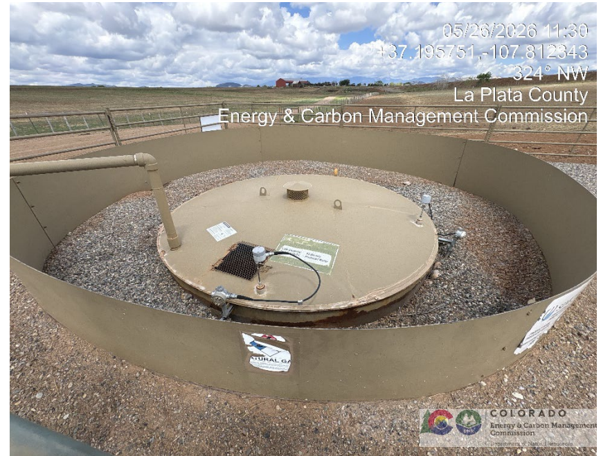
12. 95 BBL tank and secondary containment.
