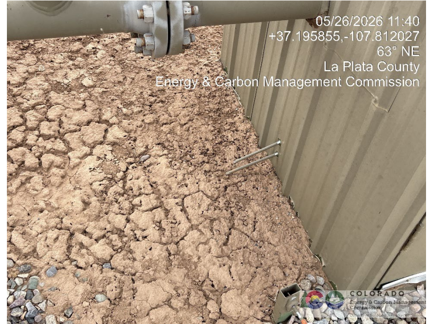
24. ¼" stainless tubes vent tubes on A4 meter shed.
