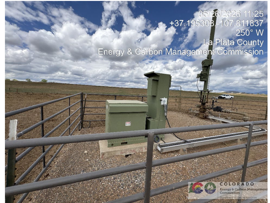
18. Linder A4 linear rod pump with electric prime mover and electrical controls behind cattle panel fence.
