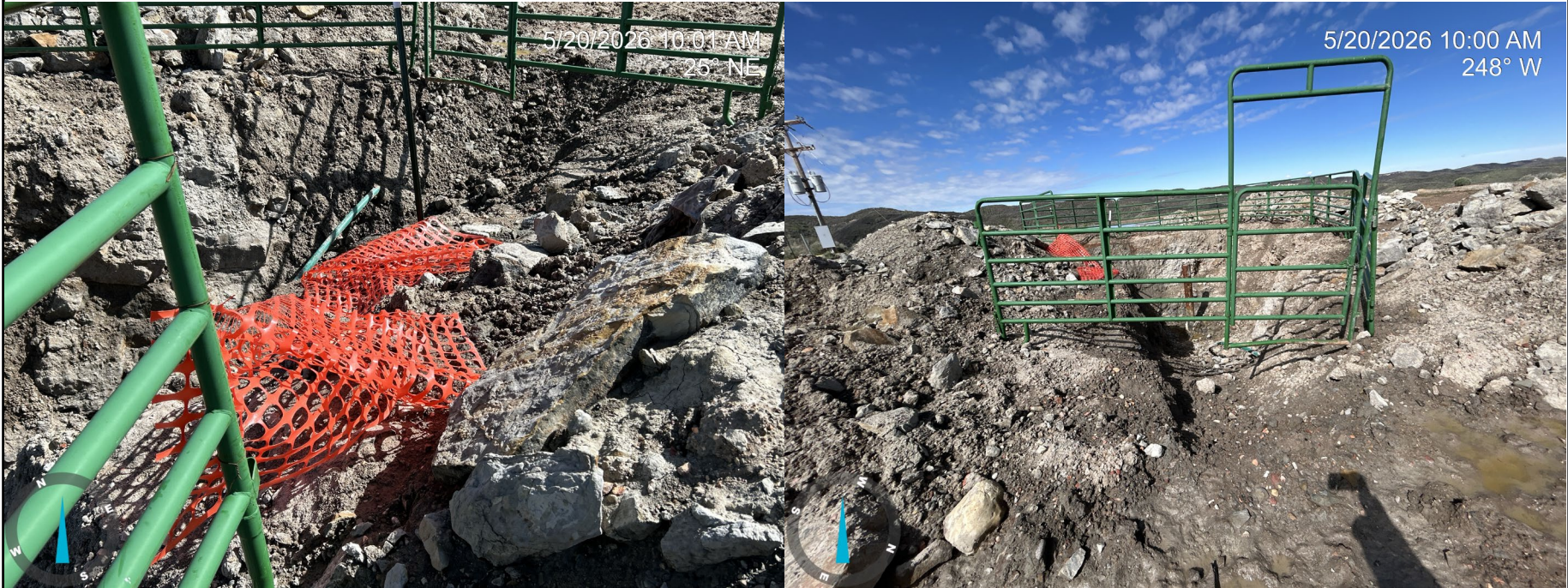
Photo 3: Photos showing orange plastic fencing around a portion of the open excavation is in disrepair and requires maintenance.
