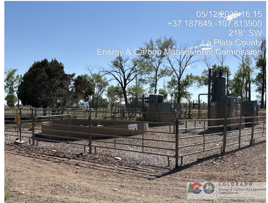
16. Produced water tank and production equipment for all wells behind cattle panel fence.
