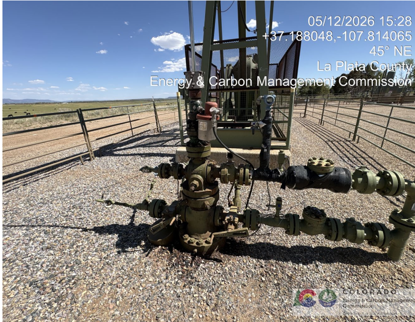
13. 15U-2R 1. De minimis staining in gravel.
