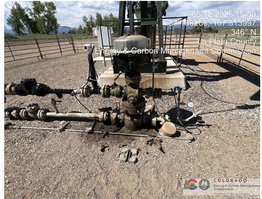
10. Well 15U-2R 3. Staining on soil near wellhead.
