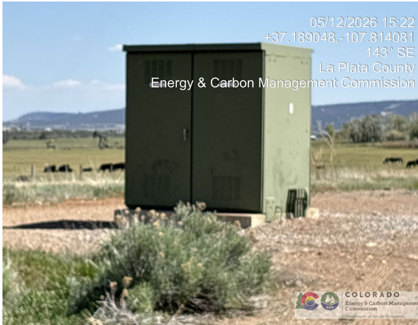
21. Electrical service near entrance gate.
