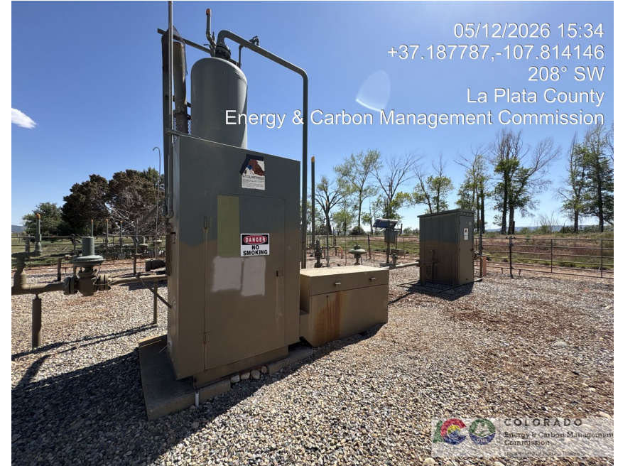
Vertical Heated Separator and Meter Run for 15U-2R 1.
