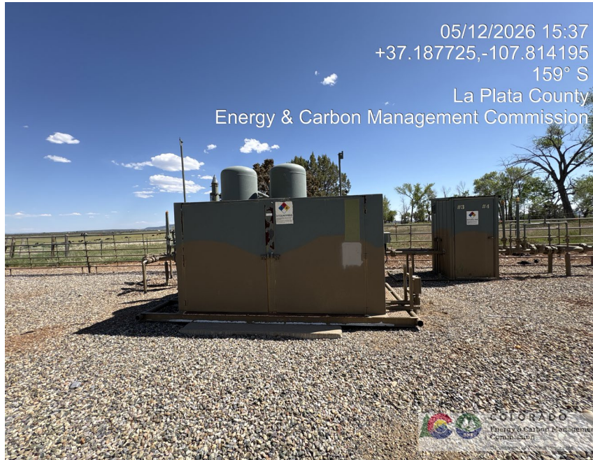
19. Vertical heated separators and meter runs for 15U-2R 3 and 15U-2R 4.
