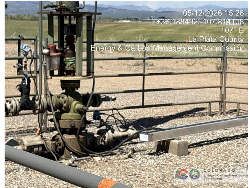
6. 15U-2R 4 wellhead. De minimis staining at base.
