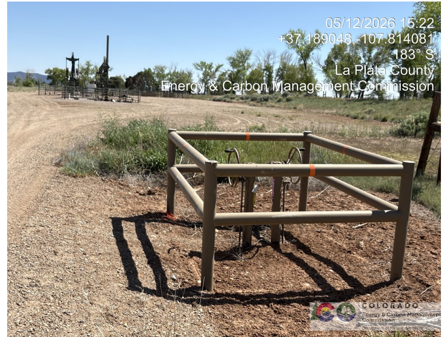
23. Flow line valve station near entrance gate.
