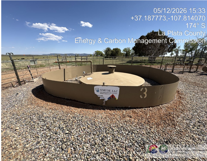
17. Steel PBV tank inside containment. Capacity 95 bbl (?). Label is peeling and illegible.
