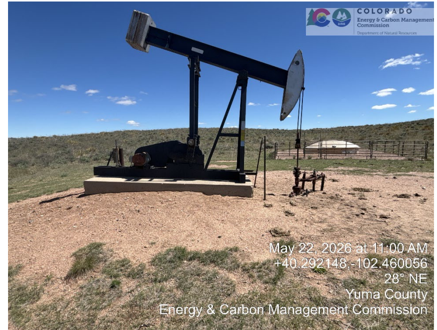
PU, Wellhead, and Tank
