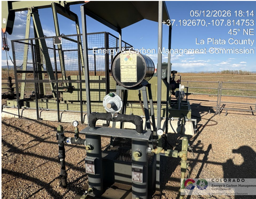
3. Lube oil container over spill prevention next to valve riser.
