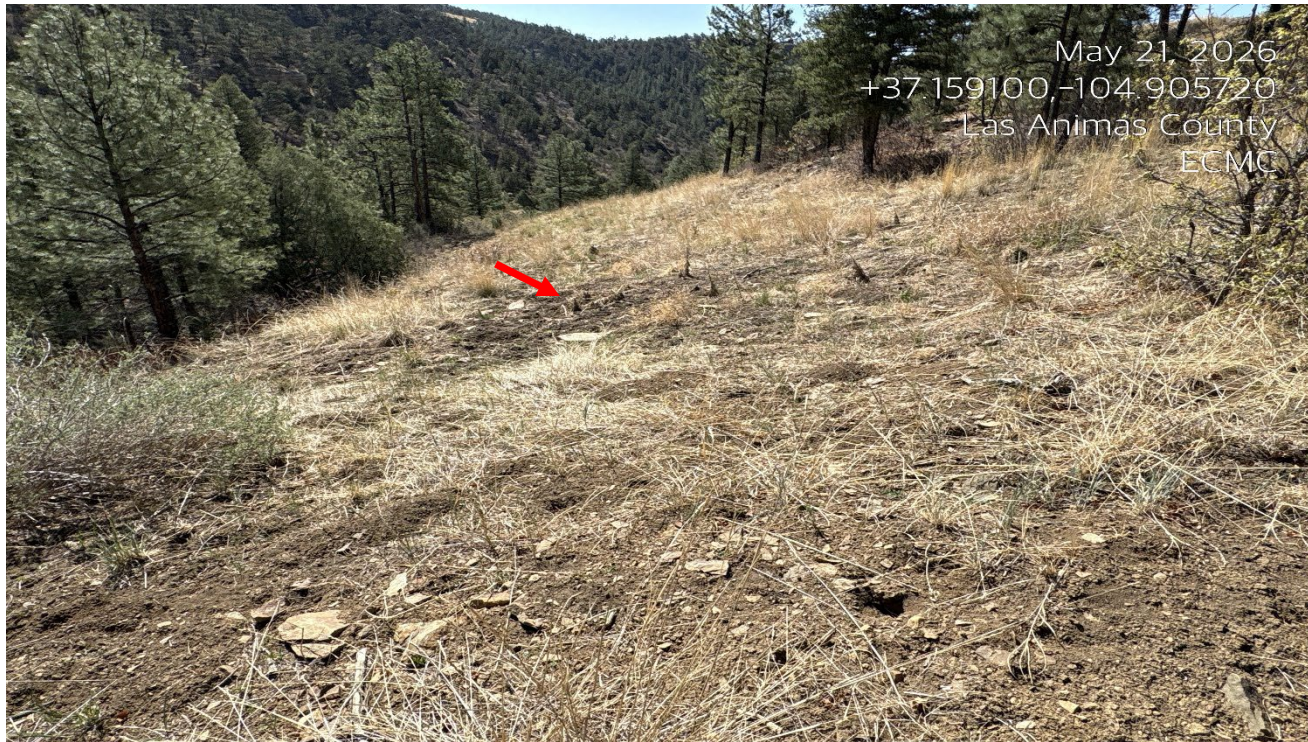
Photo 1. Facing southeast at the beginning of the reclaimed access road. There are noxious weeds emerging at red arrow that need herbicide control.
