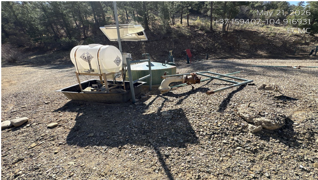
Photo 3. There are tanks and risers that don't appear to be needed or in use and must be removed.
