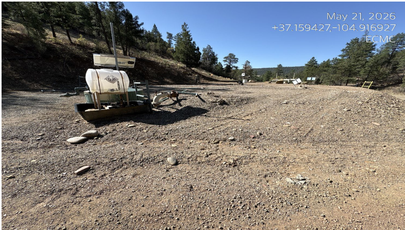
Photo 1. Facing southeast toward the GE 9 compressor station. The compressor has been removed. Unused pipe risers and equipment still remain.
