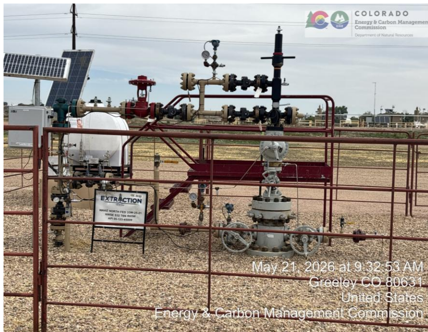
Photo 1 well head and equipment
