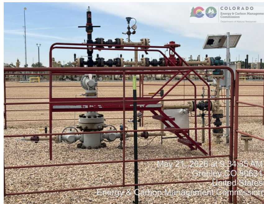
Photo 2 well head and equipment
