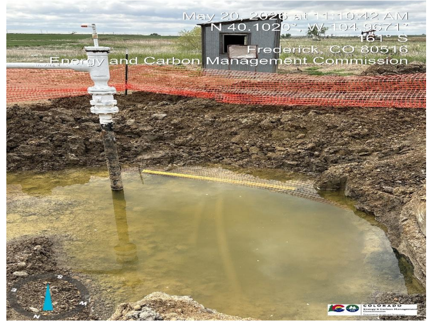
Closer view of (2) 3" fiberglass flowlines operated by KPK exposed in excavation; standing ground water in excavation.
