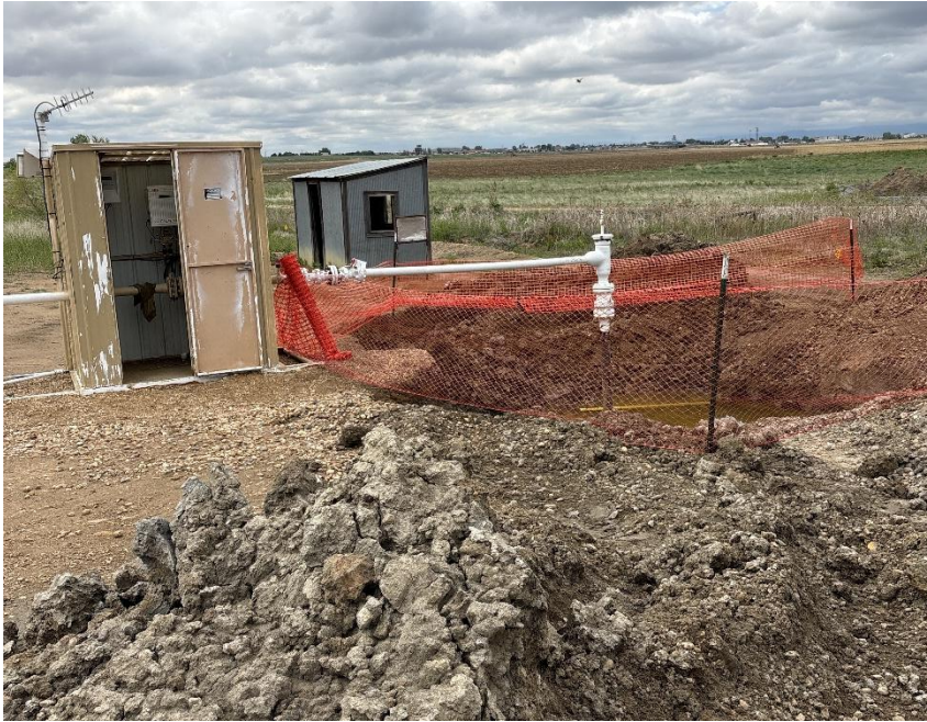
View from location looking south at fenced excavation on the west side of the Western Midstream gas meter run. The KPK outbuilding houses a flowline manifold.
