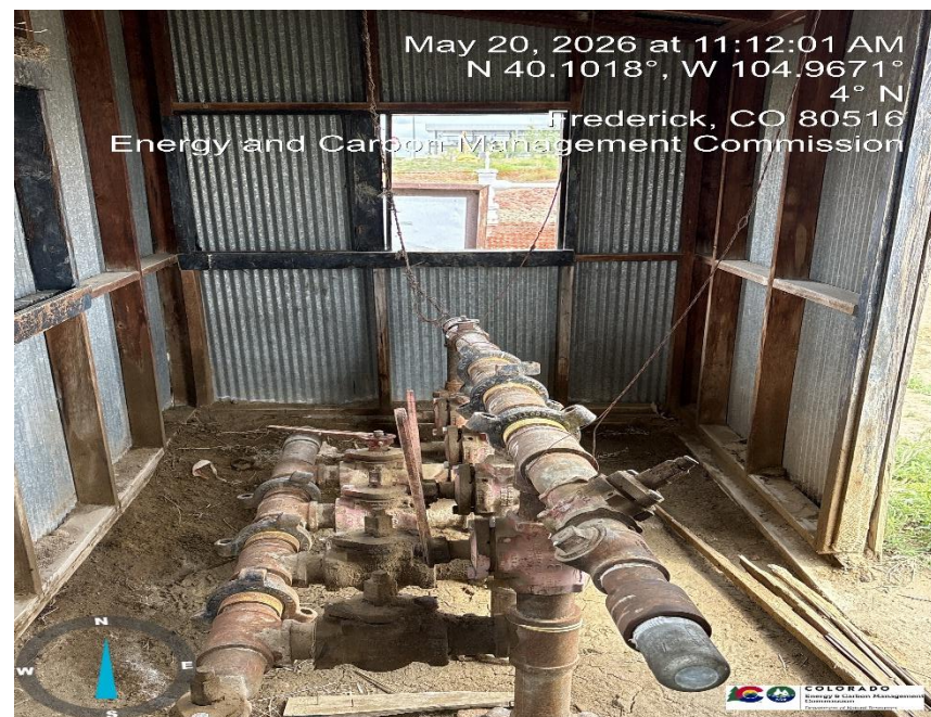
Photo of KPK Lanson Farms flowline manifold in outbuilding.
