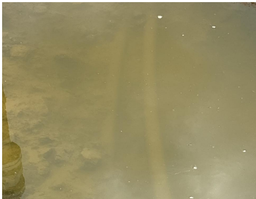
Close up view of (2) KPK 3" fiberglass flowlines unearthed in the excavation. Standing groundwater in excavation makes it difficult to see the flowlines in any detail.
