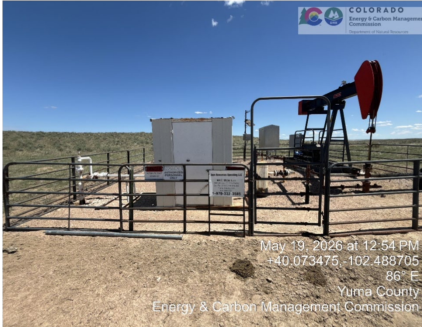
Meter run and Wellhead
