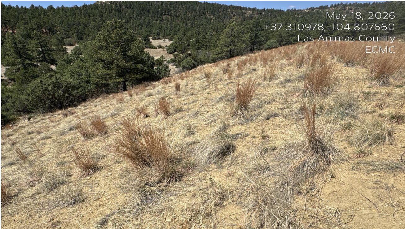
Photo 5. Facing west along the fill slope which is stabilized with desirable vegetation.
