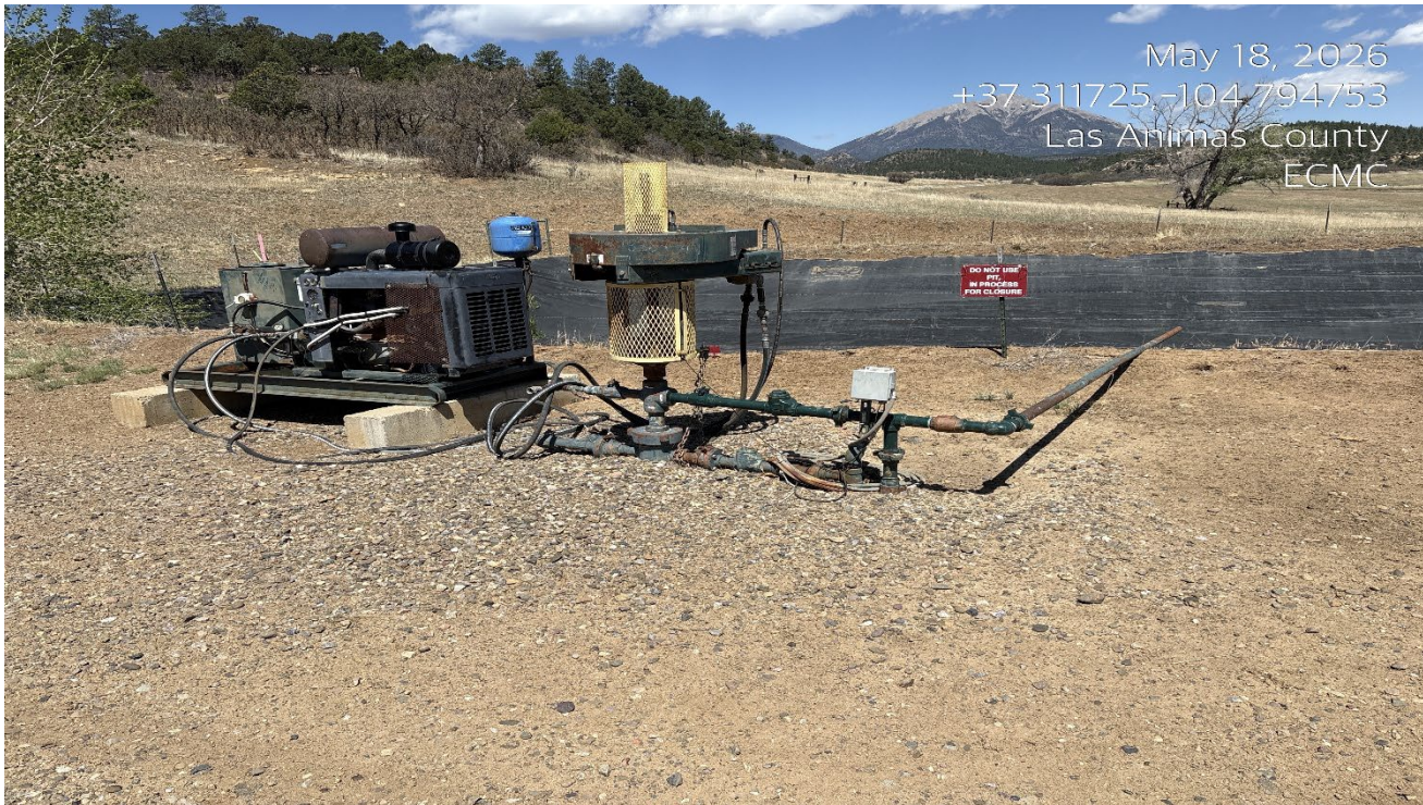
Photo 2. Facing toward the wellhead and produced water pit. Pit shows closure in process.
