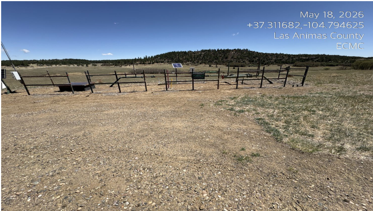
Photo 3. Well sign is posted at meter run.
