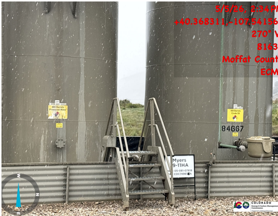
Battery signage lacks information
