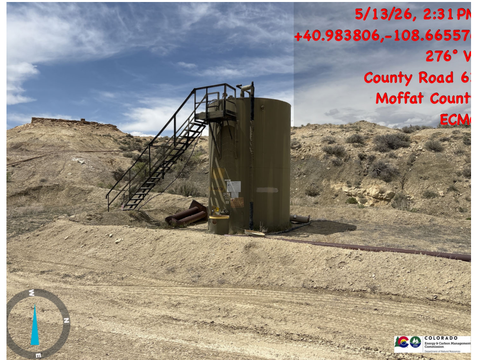
Location/ lack of battery signage
