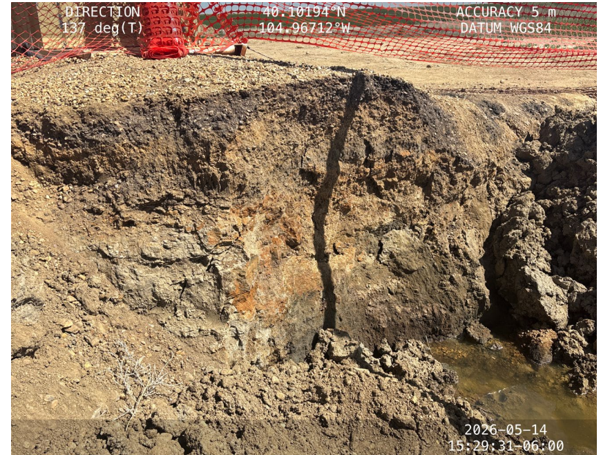
Oxidized soil along the sidewall of the excavation
