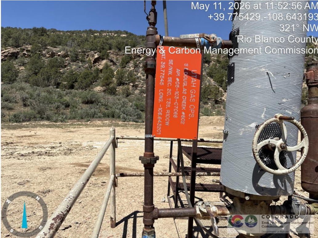
Rusty flowlines on well head.
