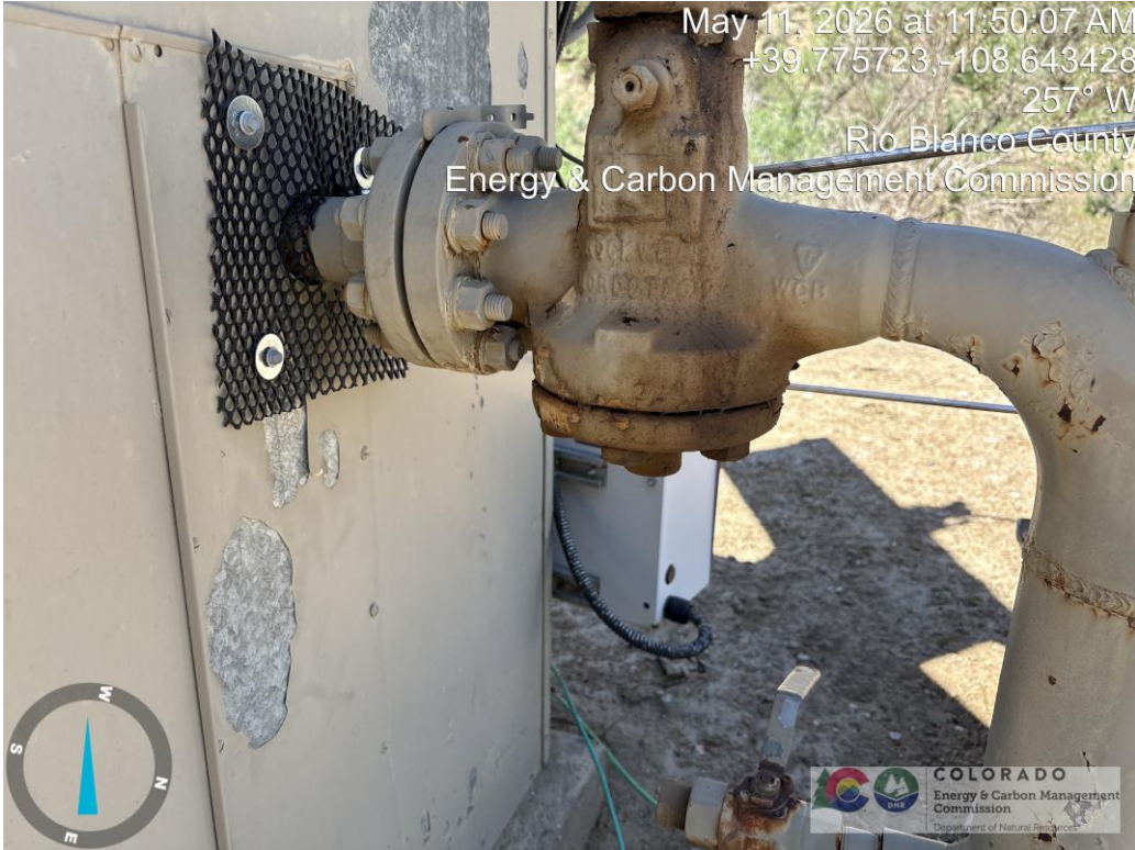
Oily residue on valve.
