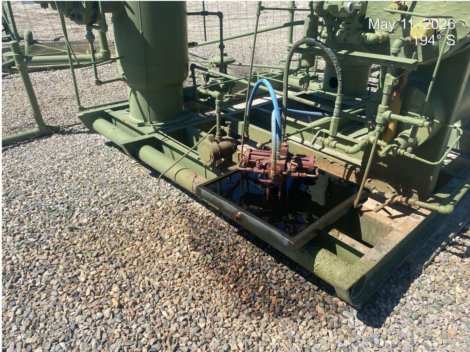
Photo 4. View of spill pan which is overflowing.
