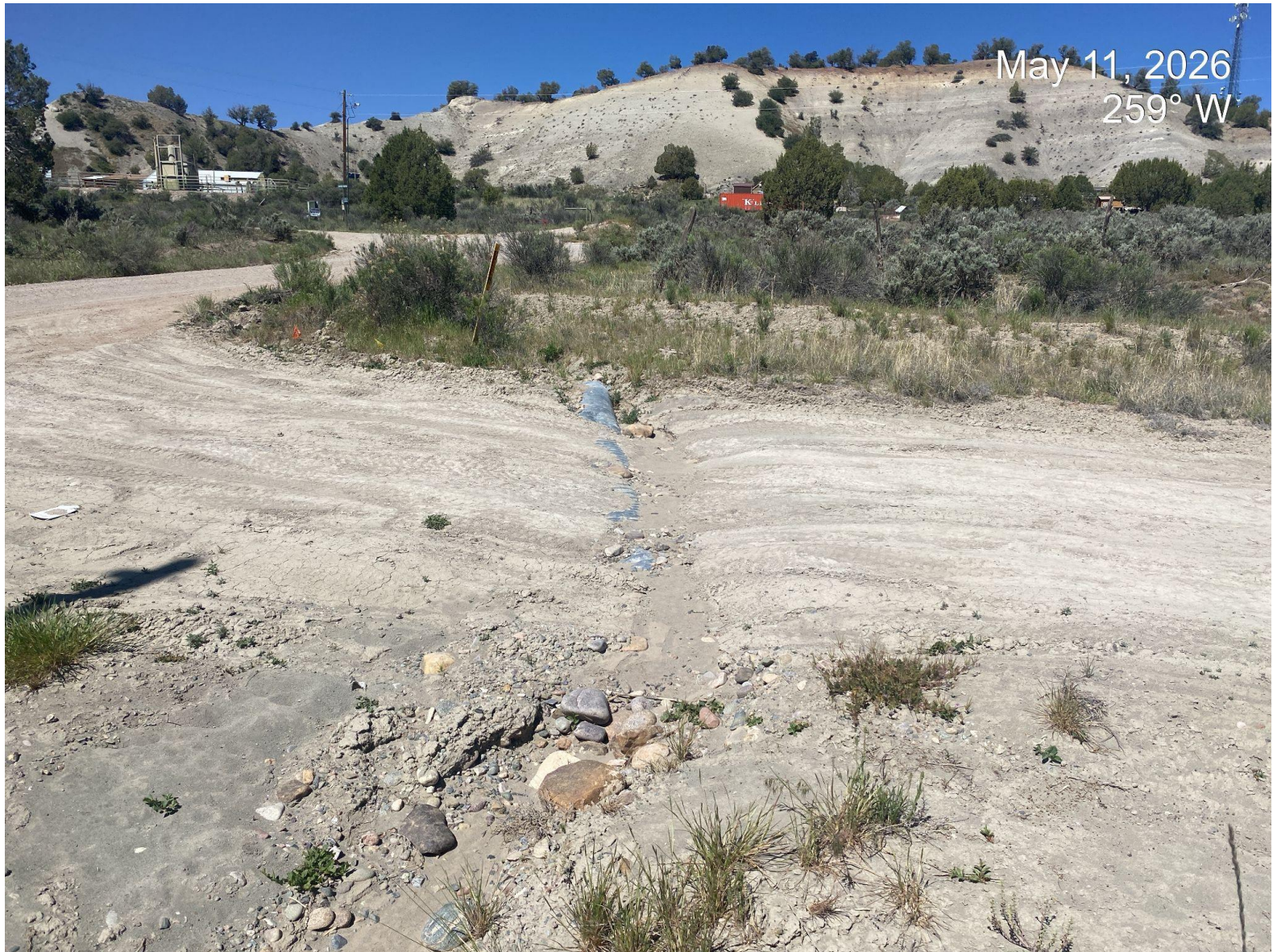
Photo 3. View of exposed culvert at access point which is crushed and no longer functioning.
