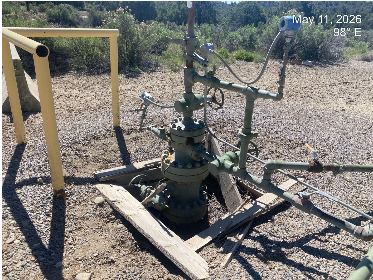
Photo 2. View of wellhead assembly equipment.
