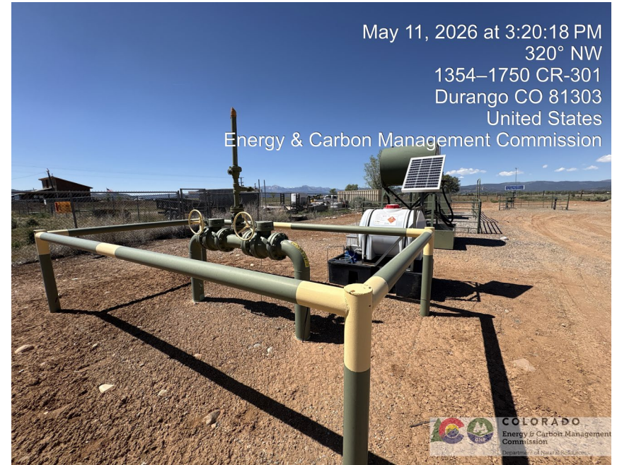
6. Valve on 6" pipeline for offsite gathering or produced water for injection well. Chemical treatment container on top of spill release with solar telemetry. Has manufacturer labelling.
