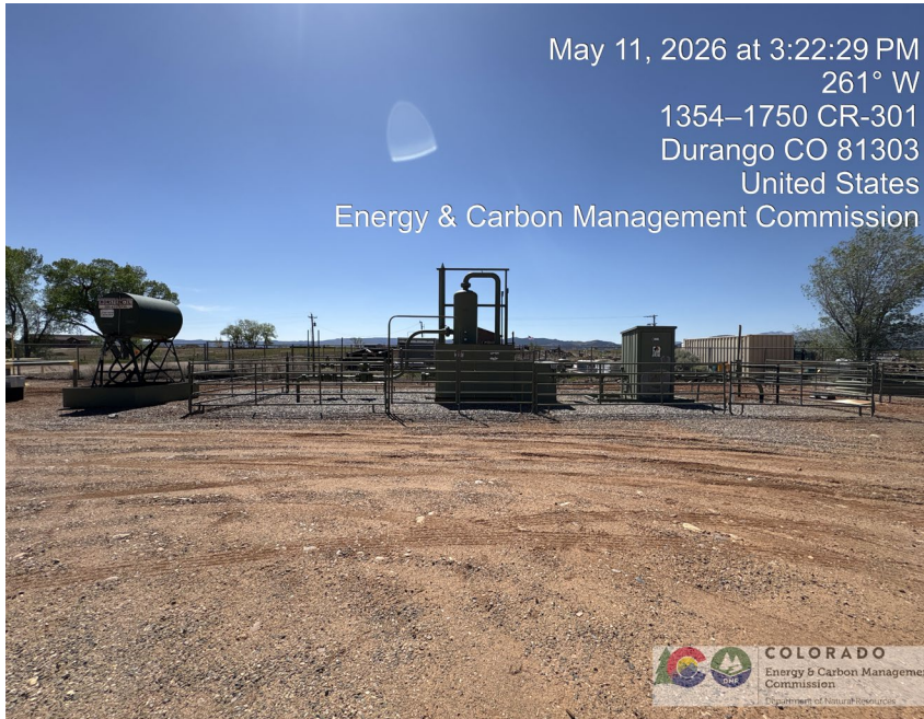
9. 15U-2R 2 production equipment behind cattle panel fence. Vertical heated separator and meter run. 4" production flowlines connecting equipment.
