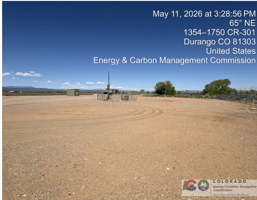
15. Location overview photo. 15E-2R 2 wellhead in middle of photo. Disposal well shelter to left. Disposal well equipment in background.
