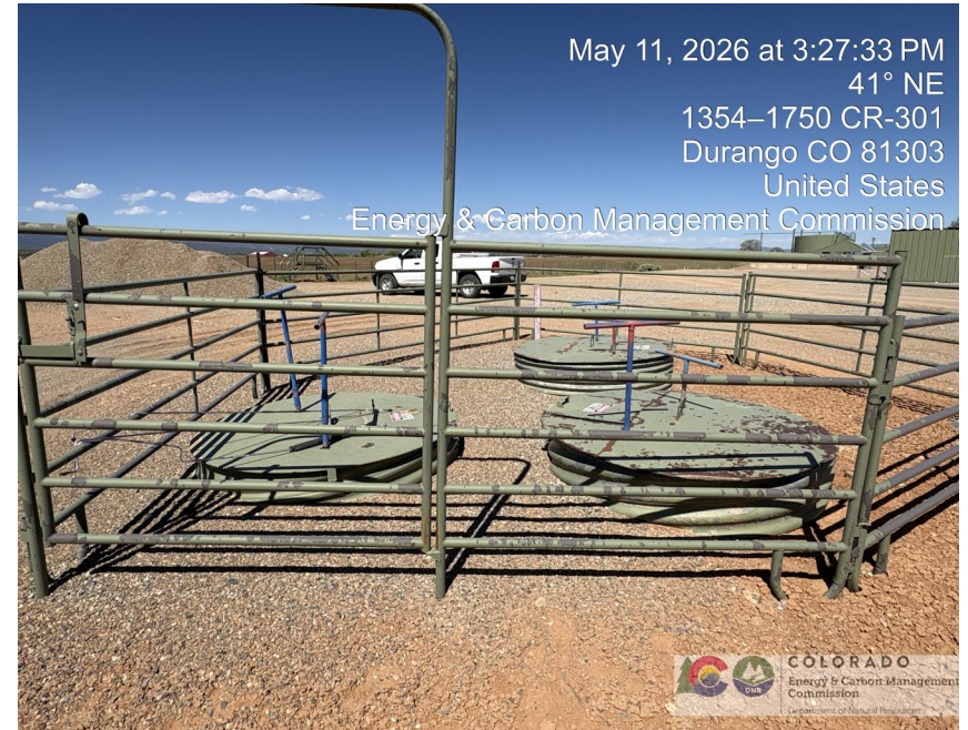
14. Three underground flow line valve access boxes with T handles.
