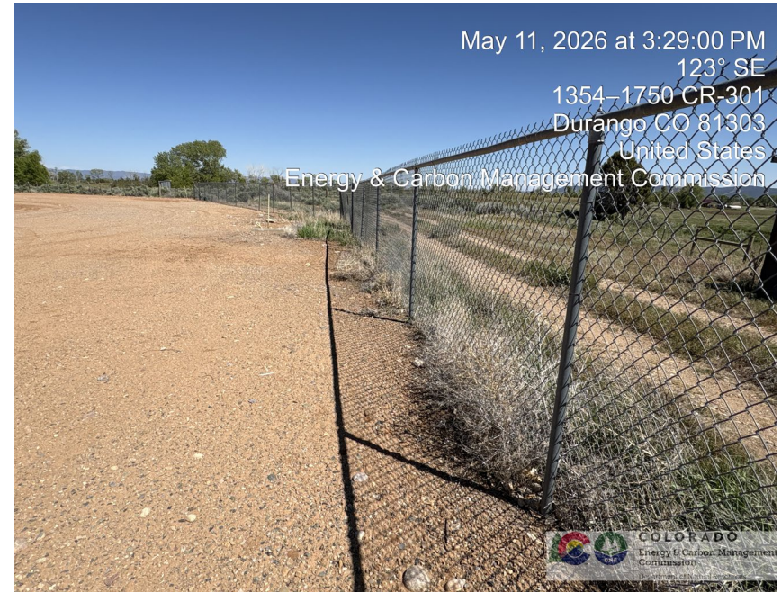
16. Location perimeter chain link fence on south side of location looking east.
