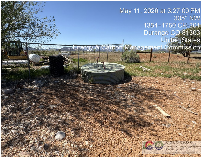
13. Underground flow line valve access box with T handle.
