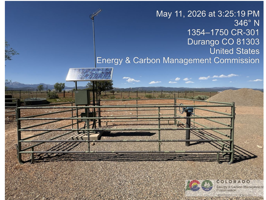
10. Solar telemetry and valve riser behind cattle panel.
