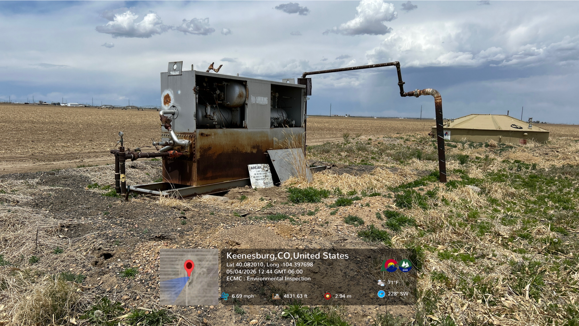
Panels on the side of the separator have been removed.
