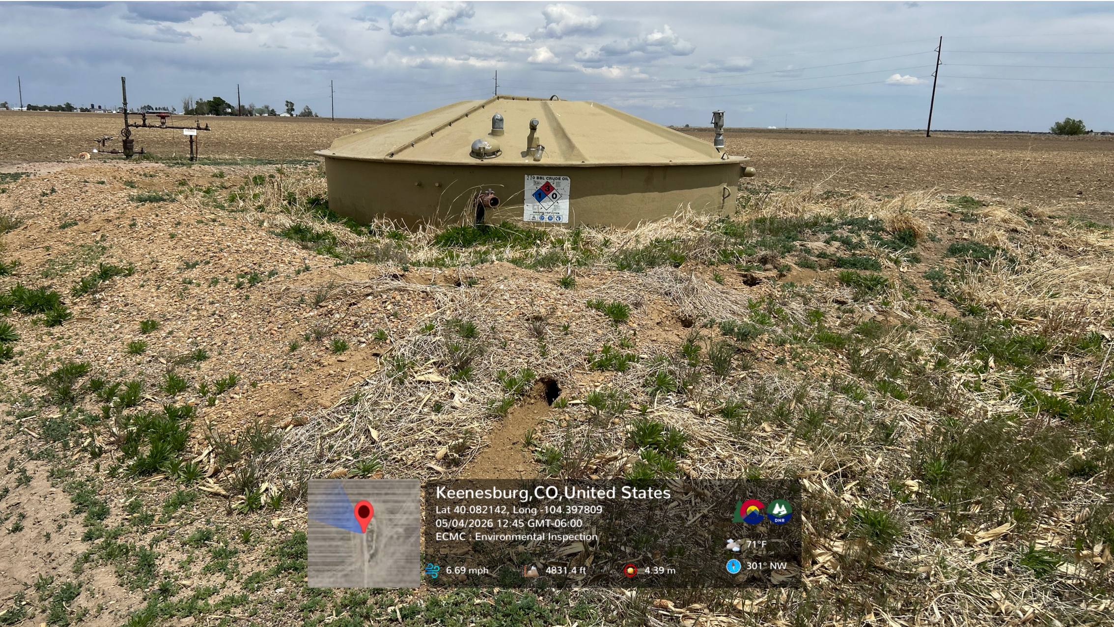
Looking at a partially buried fiberglass tank (foreground). Multiple holes/burrows are visible in the tank containment berm.
