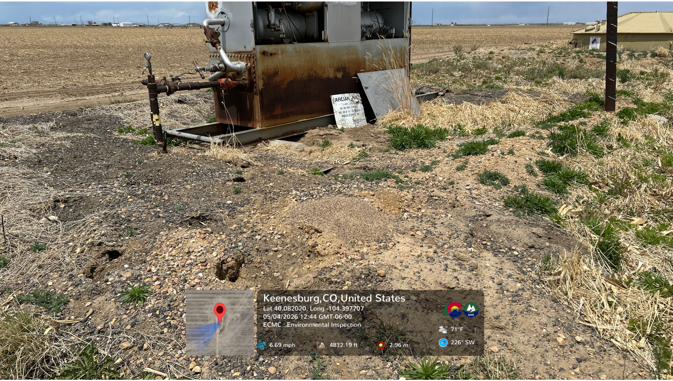
Multiple holes/burrows are visible in the separator containment berm. The berm material fails when walked on.
