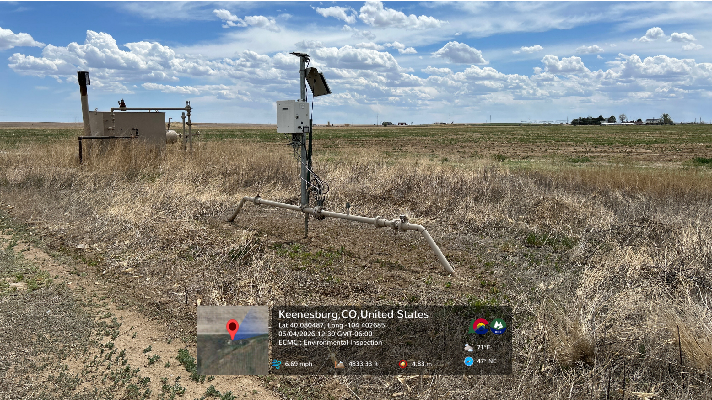
Looking at separator and meter station.
