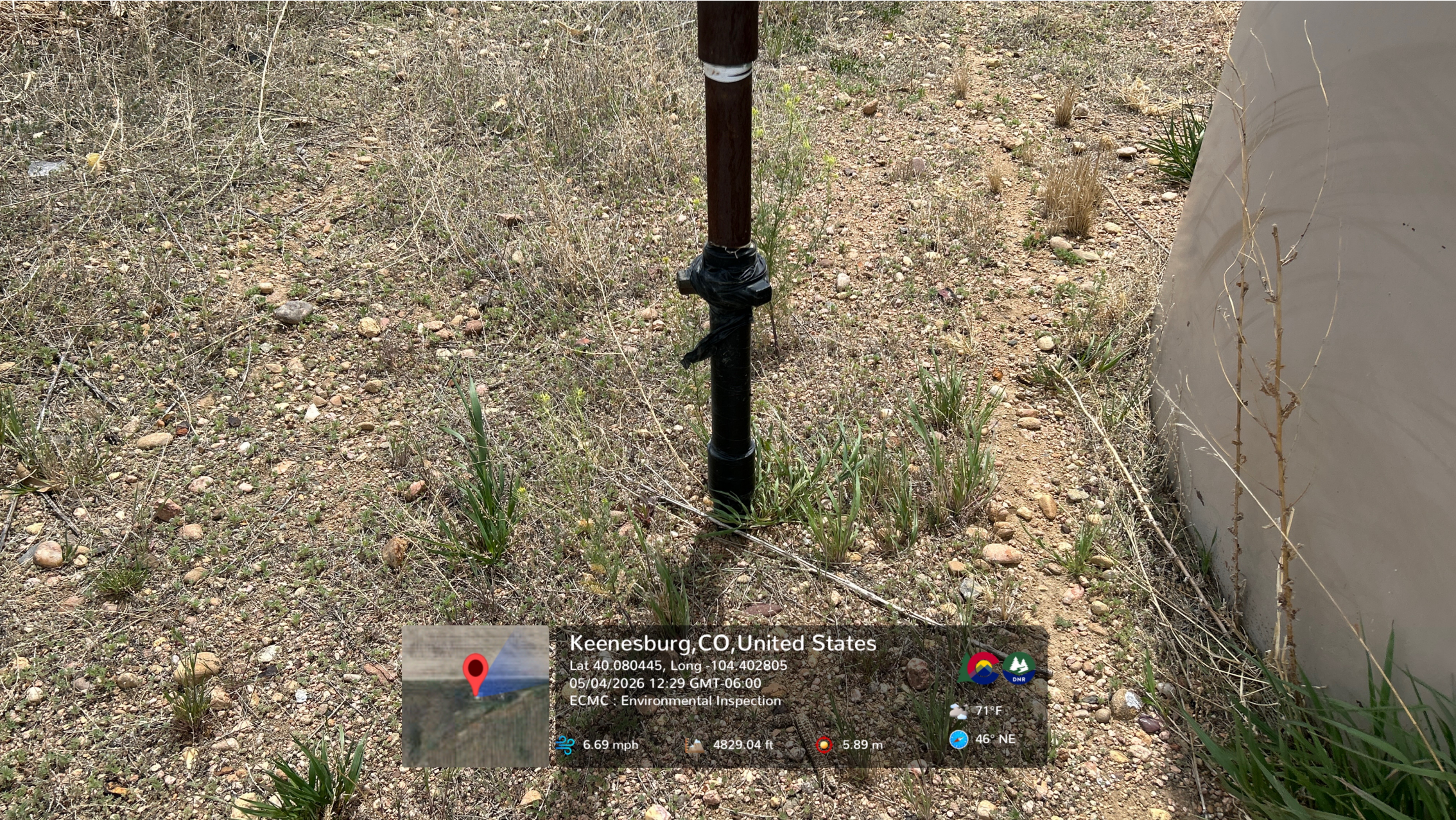
Black tape is wrapped around a portion of riser adjacent to the crude oil AST.
