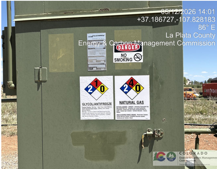
7. Labels on separator access hatch.
