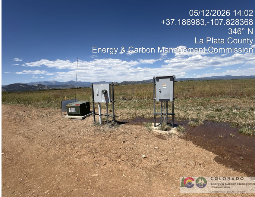
9. Electrical service panels on north edge of pad. Area is wet from irrigation water from off location.
