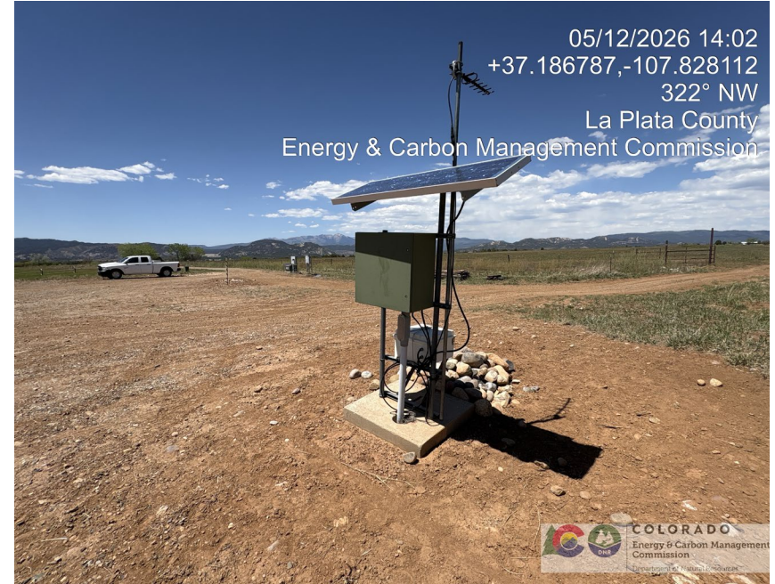
10. Solar telemetry. Electrical service panels from photo 9 in distance.
