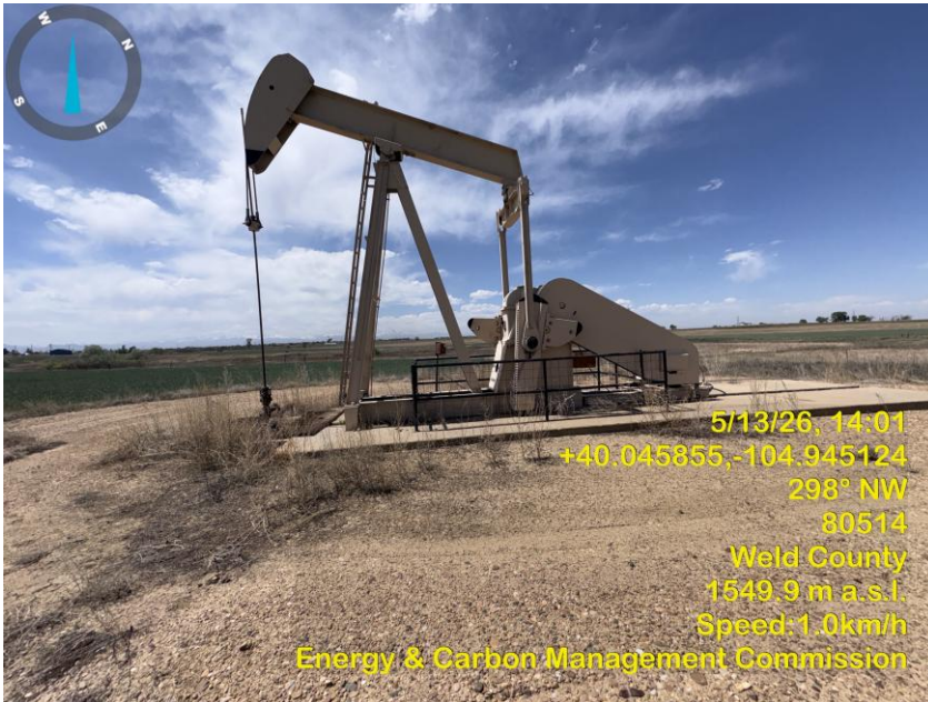
Photo 7 Wellhead sign is faded.
