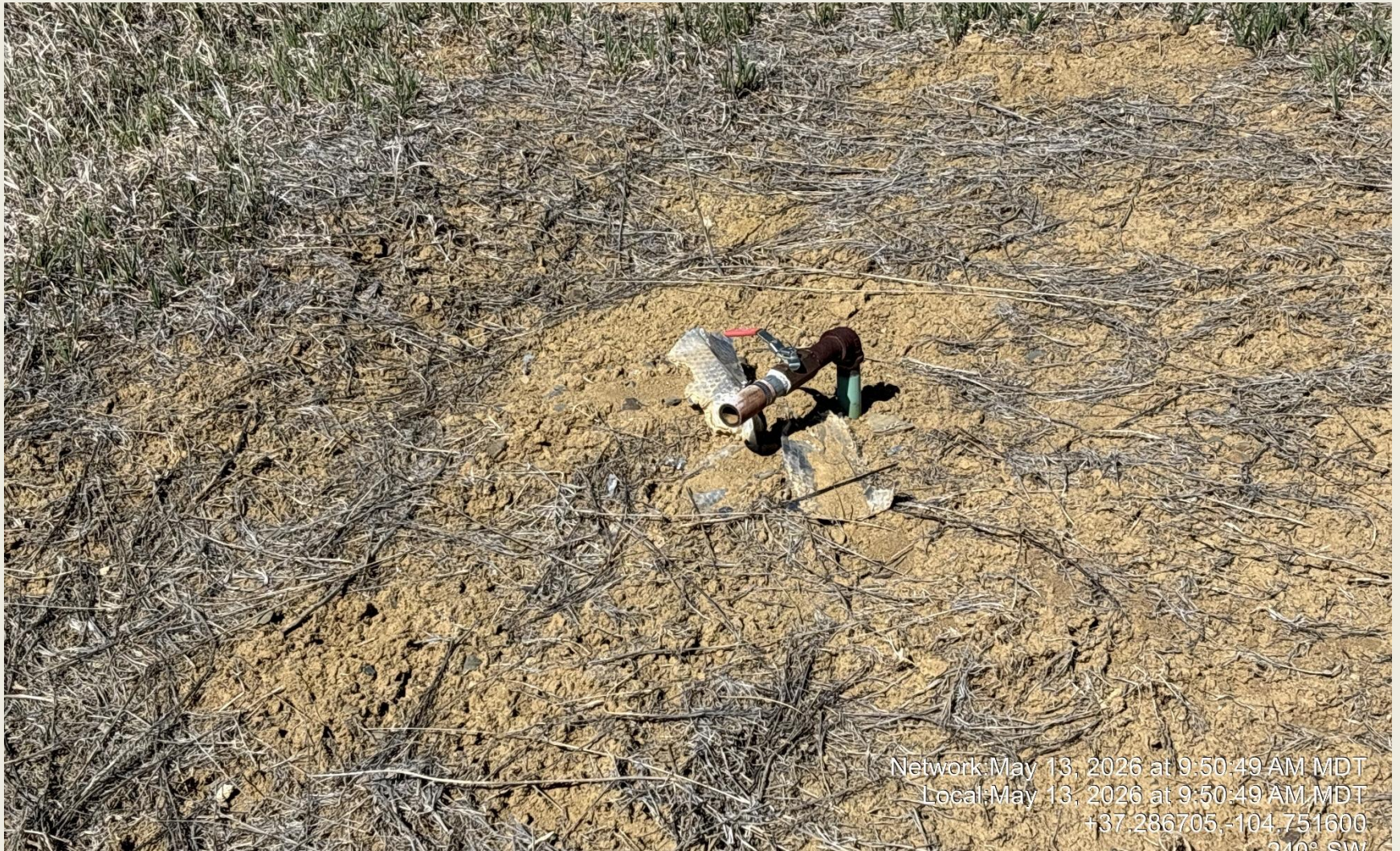
PHOTO 7: UNUSED EQUIPMENT (1" RISER NEAR WELLHEAD NOT LABELED). REMOVE OR LABEL RISERS PER RULE 606. CA DATE 6/13/2026.
