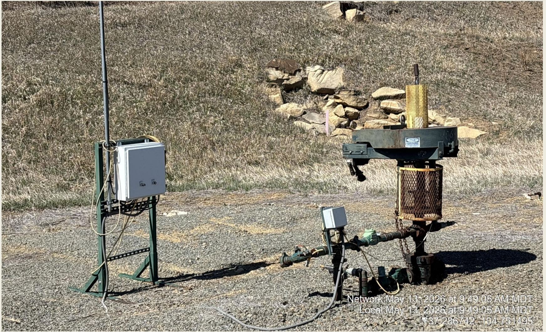
PHOTO 4: WELLHEAD AND EQUIPMENT.
