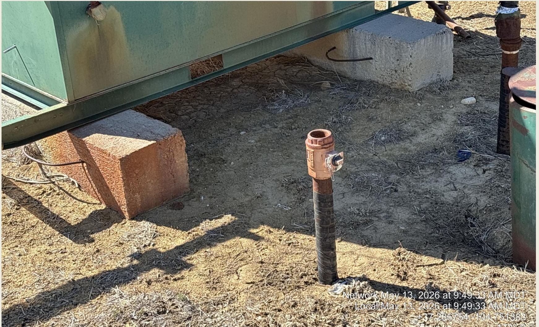
PHOTO 5: UNUSED EQUIPMENT (2" RISER NEAR METER HOUSE NOT LABELED). REMOVE OR LABEL RISERS PER RULE 606. CA DATE 6/13/2026.
