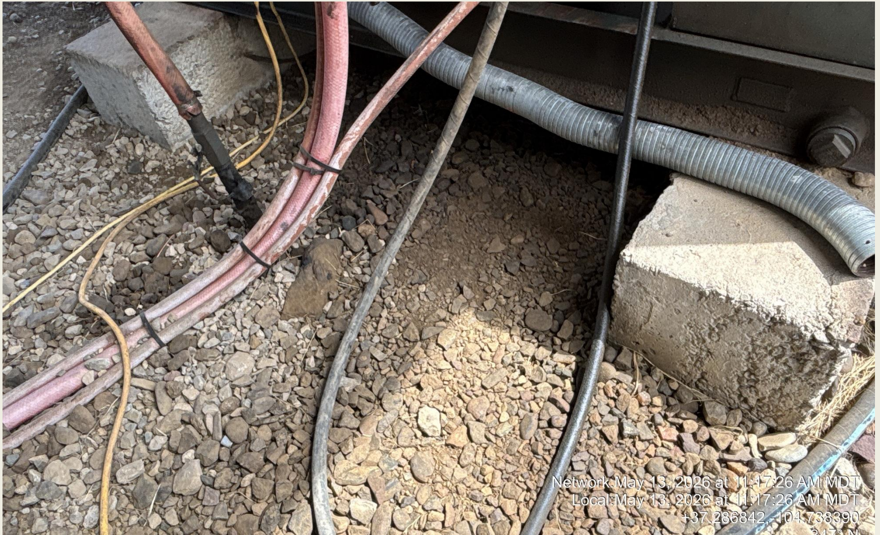
PHOTO 6: AREA OF IMPACTED SOIL NEAR PRIME MOVER SKID. AT TIME OF INSPECTION THIS EQUIPMENT IS NOT IN OPERATION HOWEVER IT APPEARS TO HAVE SIGNIFICANT OIL LEAKS THAT SHOULD BE REPAIR PRIOR TO PUTTING EQUIPMENT BACK IN USE. Conduct maintenance on equipment, cleanup stained material and review self inspection processes. COMPLY WITH RULE 1002,(2).D CA DATE 6/13/2026.
