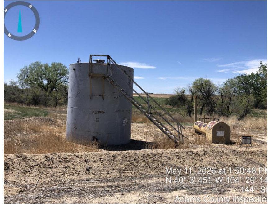
Photo #2 Tank & separator.
