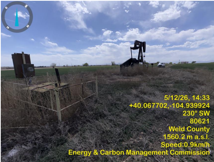
Photo 7 Dead vegetation around wellsite.
