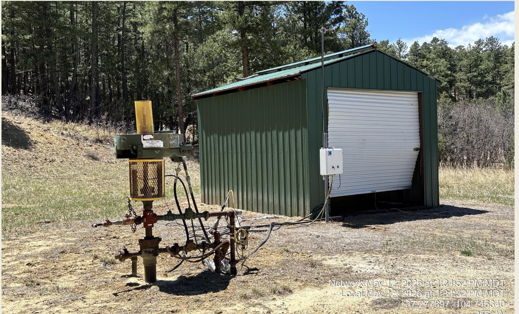
PHOTO 5: TR WELLHEAD AND EQUIPMENT.
