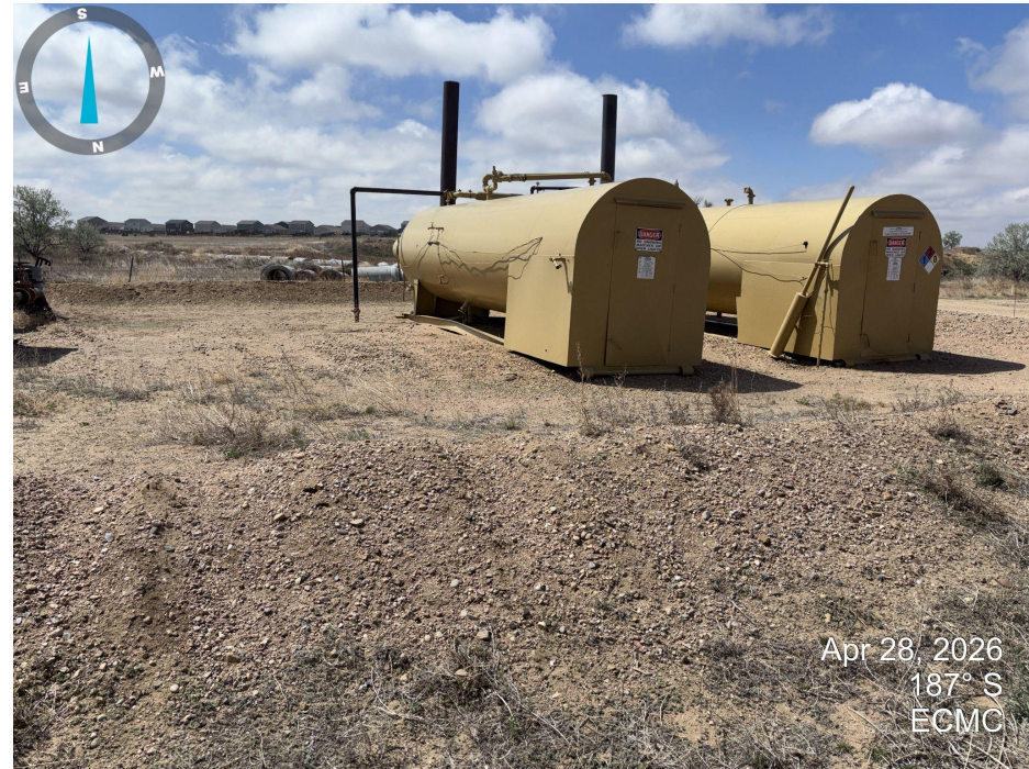
Photo 6. Separators on location inside secondary containment.
