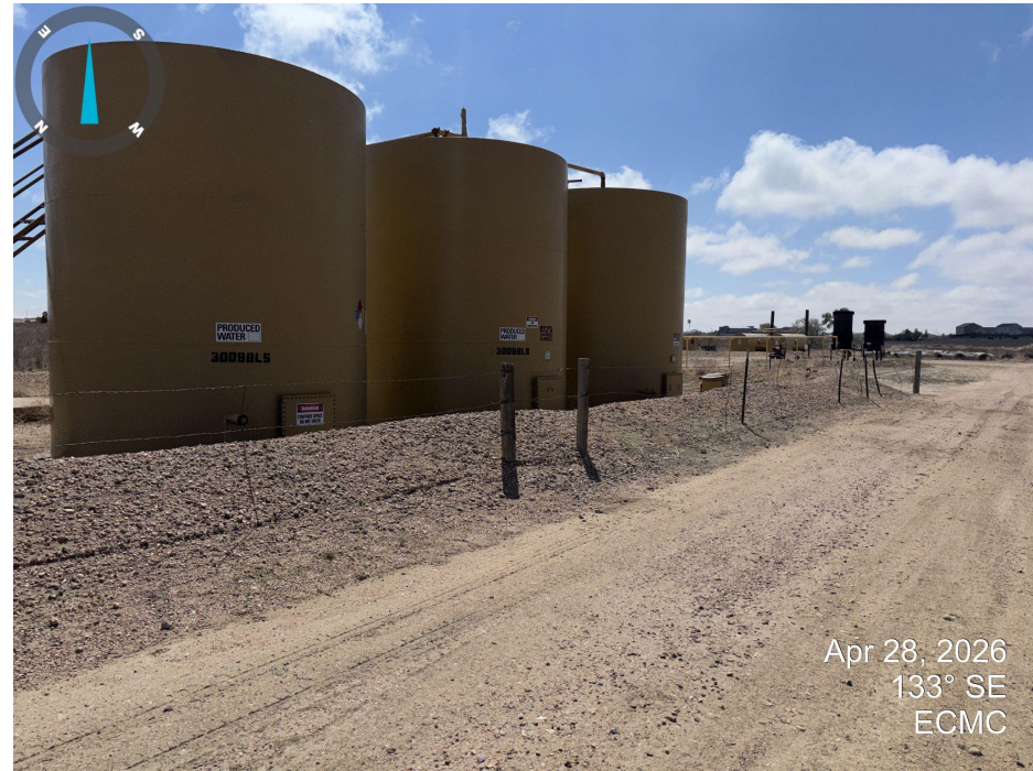
Photo 8. Storage tanks on location.
