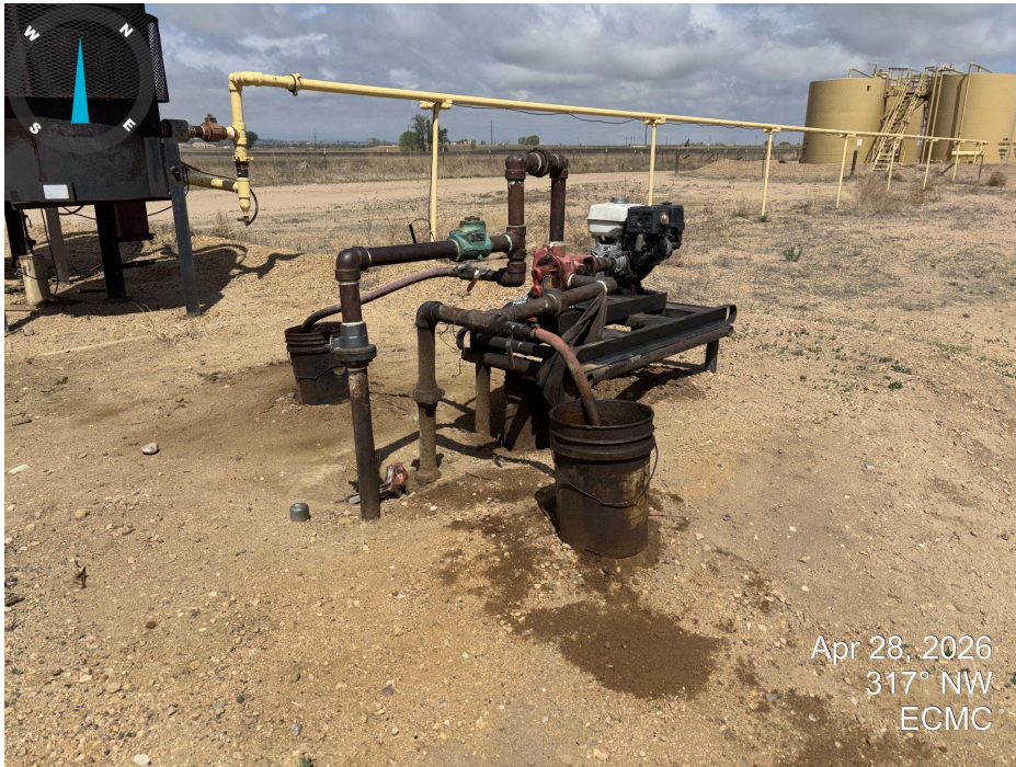
Photo 3. Photo taken at small pump assembly near VCDs. Stained soil is present around pump. Dark fluid was observed in three buckets around the pump. Leaking fittings were observed on the pump.
