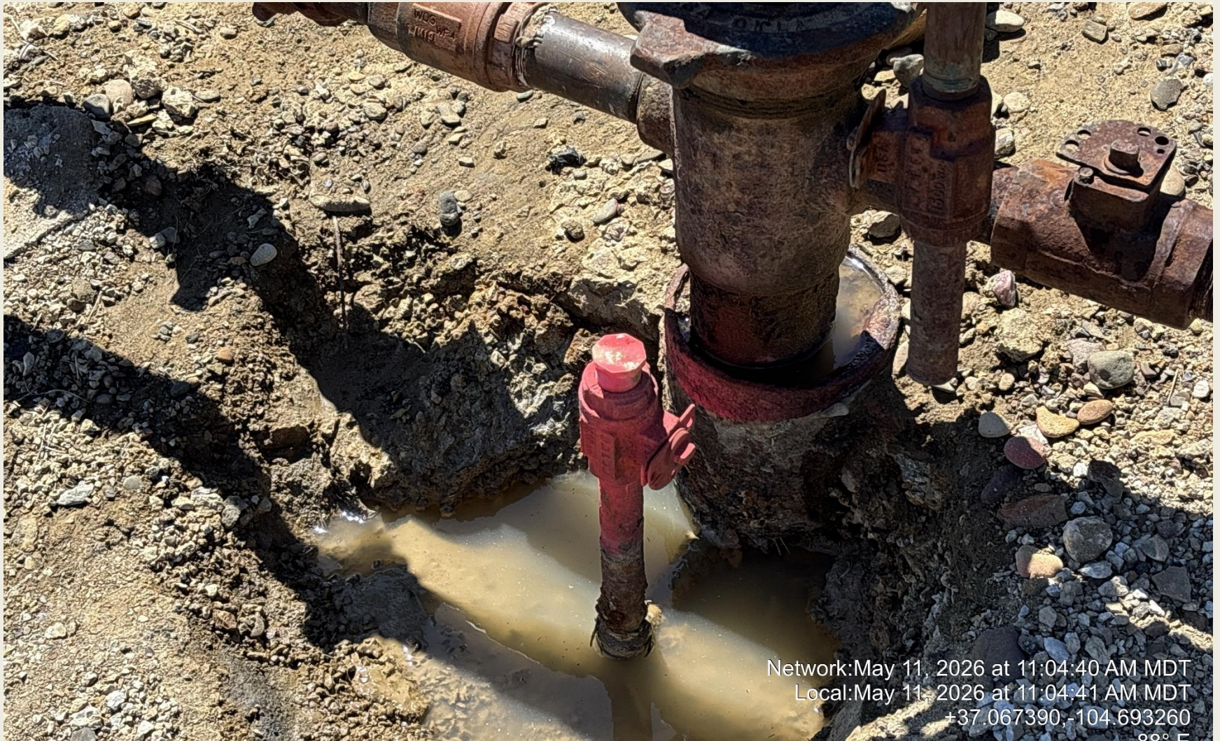
PHOTO 5: SURFACE CASING IS TOPPED OFF WITH WATER AND THERE ARE NO GAS BUBBLES.
