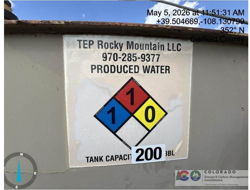
Photo # 6135 Tank capacity incorrect
