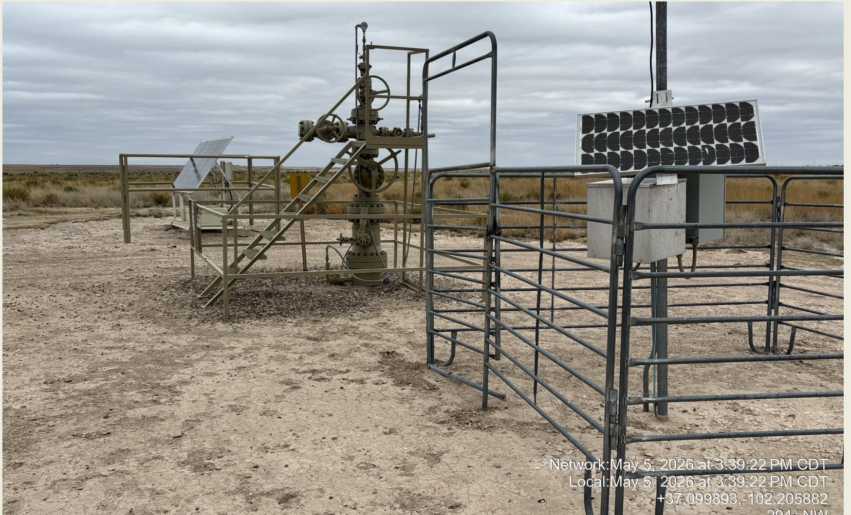
PHOTO 4: WELLHEAD AND EQUIPMENT.
