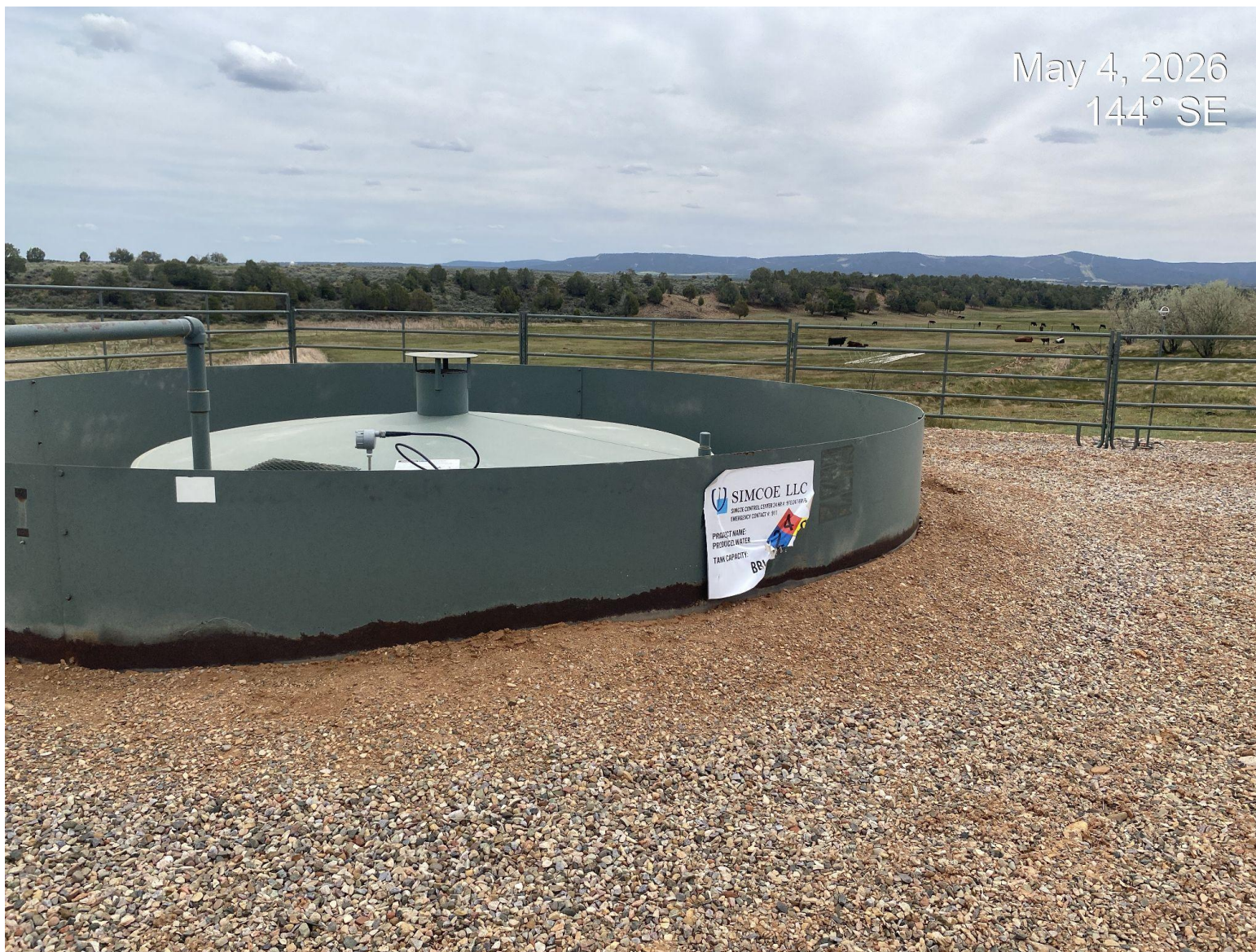
Photo 4. Produced water tank label is peeling and no longer legible.
