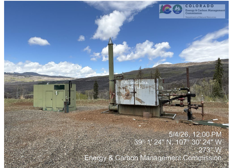
Separator and Generator
