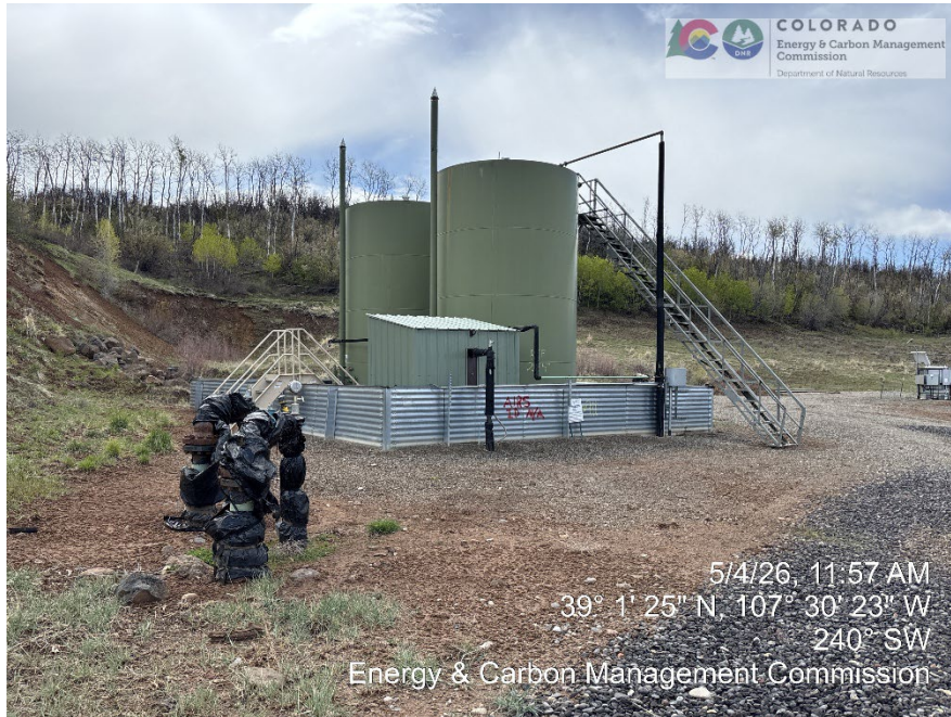
Off location flowline risers
