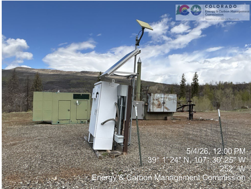
Electrical Control panel
