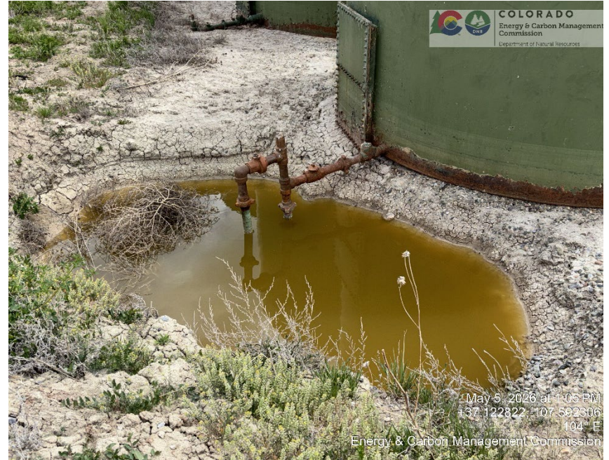
POSSIBLE FLOW LINE LEAK
