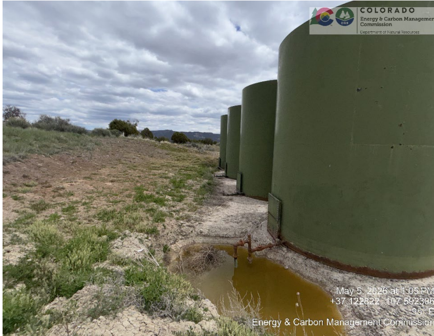
POSSIBLE FLOW LINE LEAK
