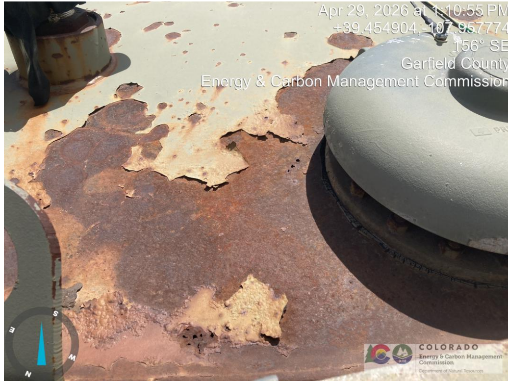
Rusted pin holes on top of tank.
