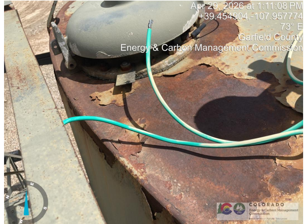
Rusted pin holes on top of tank.
