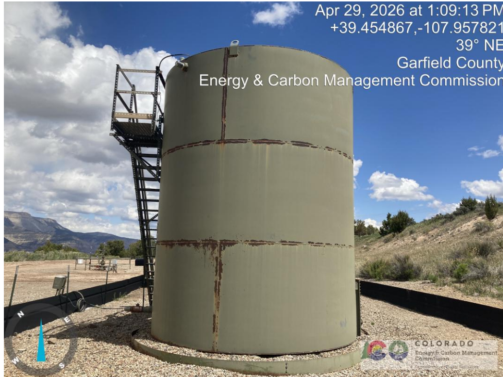
Tank rusted around seams.
