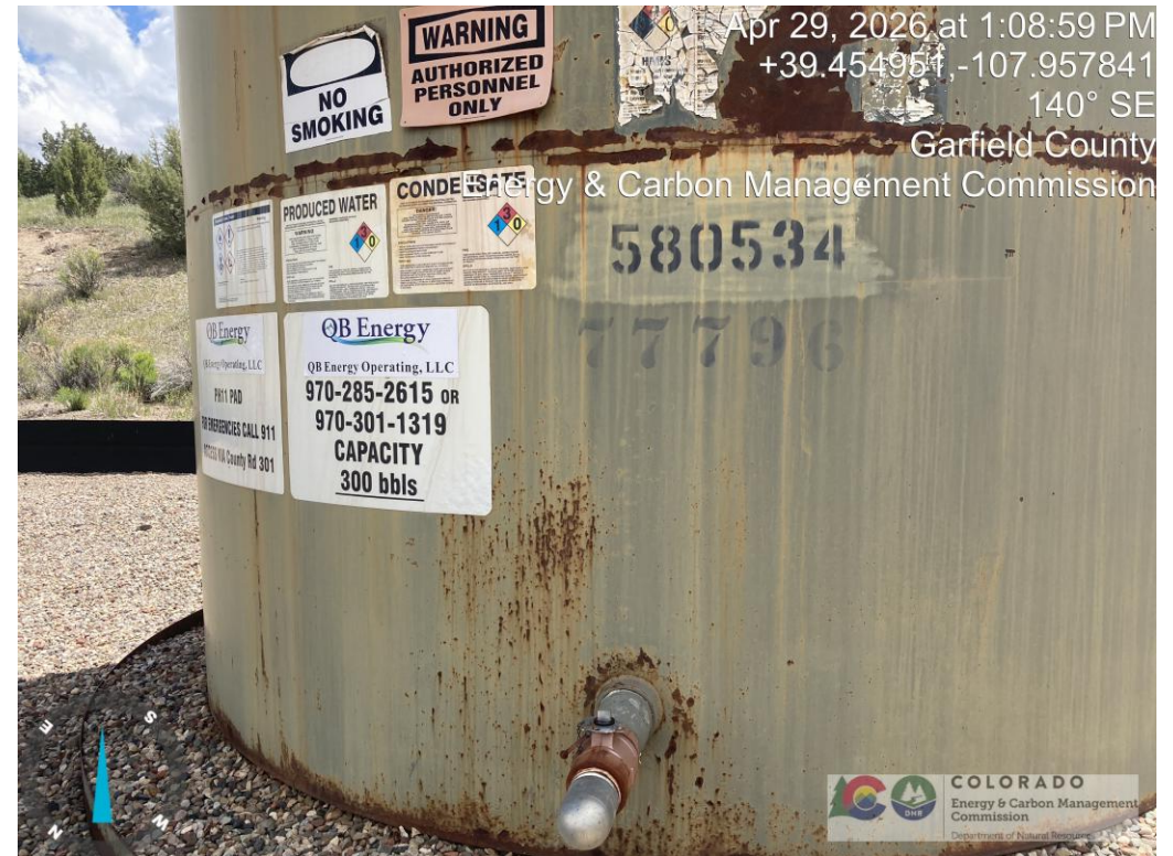
Rusted pinholes around bottom tank valve.
