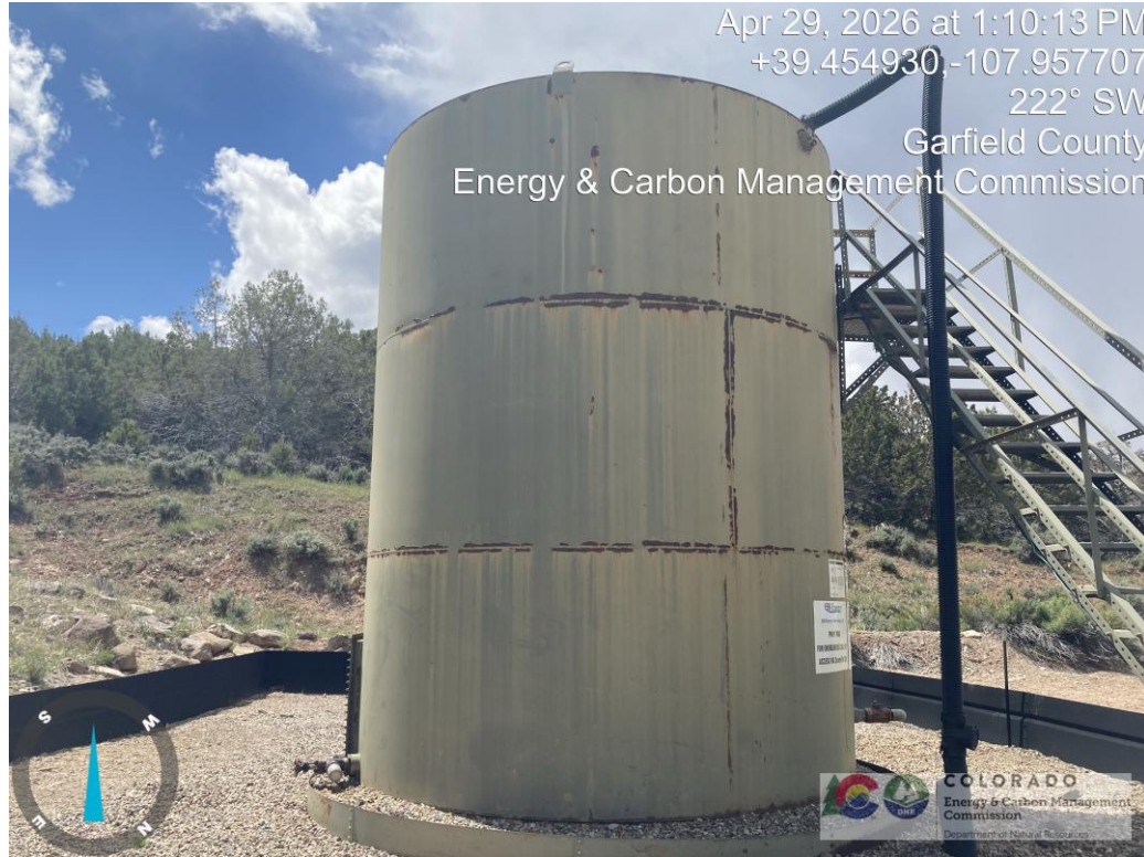
Tank rusted around seams.
