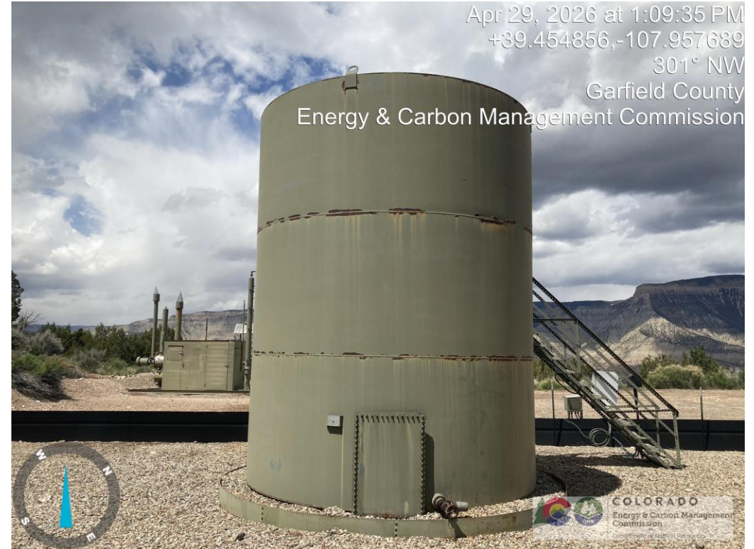
Tank rusted around seams.
