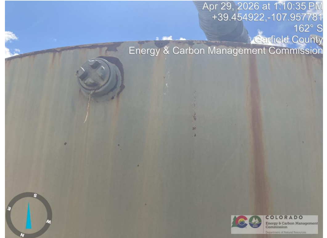
Tank top seam rusted through.
