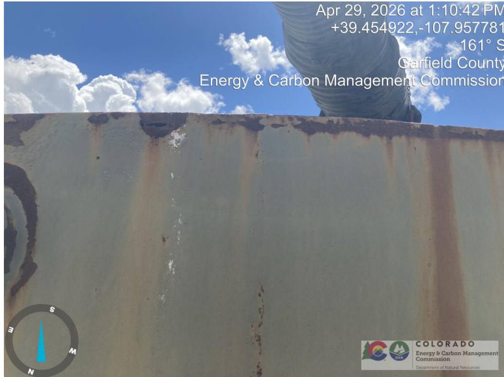
Tank top seem rusted through.
