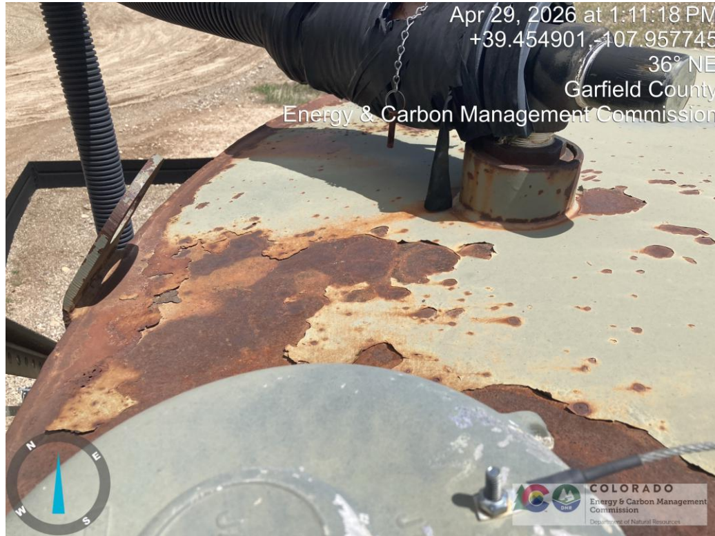
Rusted pin holes on top of tank.
