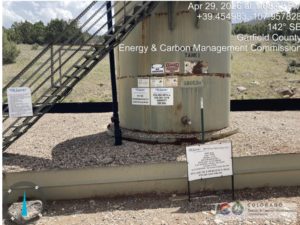
Tank rusted around seams.
