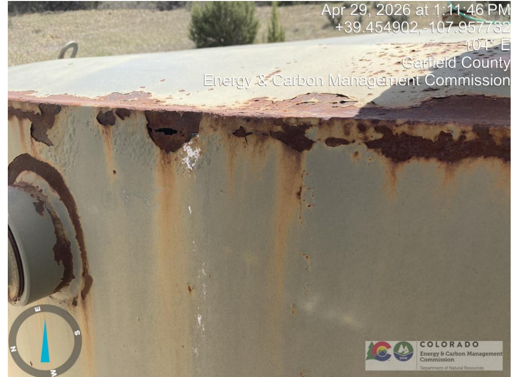
Tank top seem rusted through.
