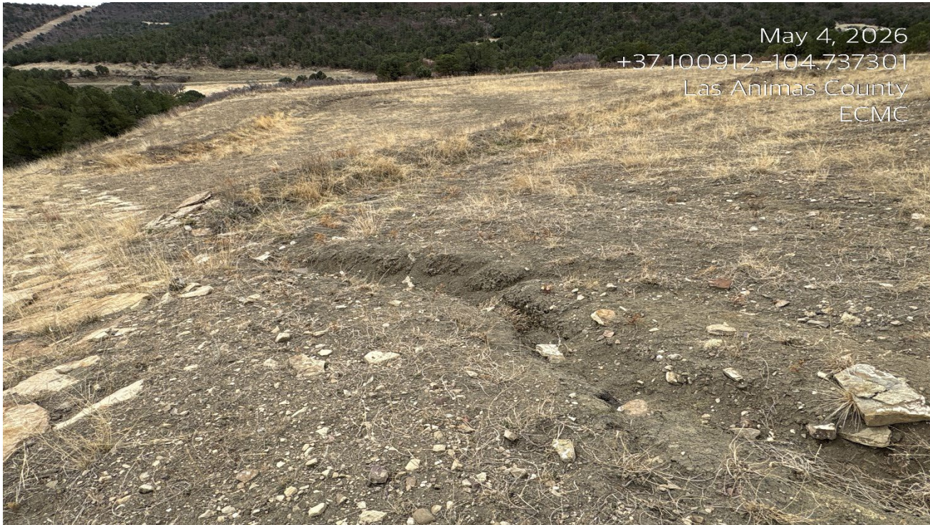
Photo 3. Facing southeast. There is an erosion channel and additional seeding should be performed.
