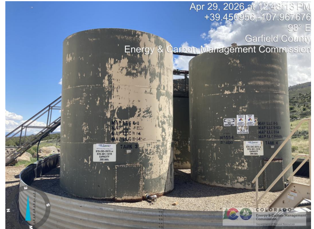
Paint deterioration and areas of rust.
