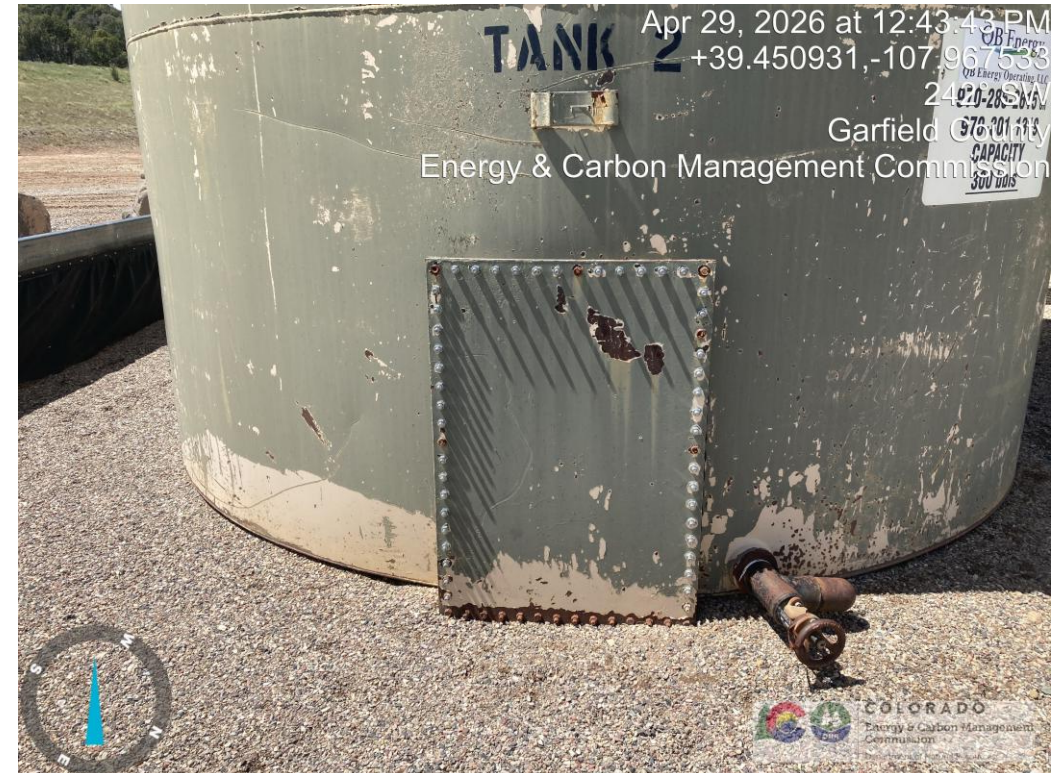
Paint deterioration and areas of rust.
