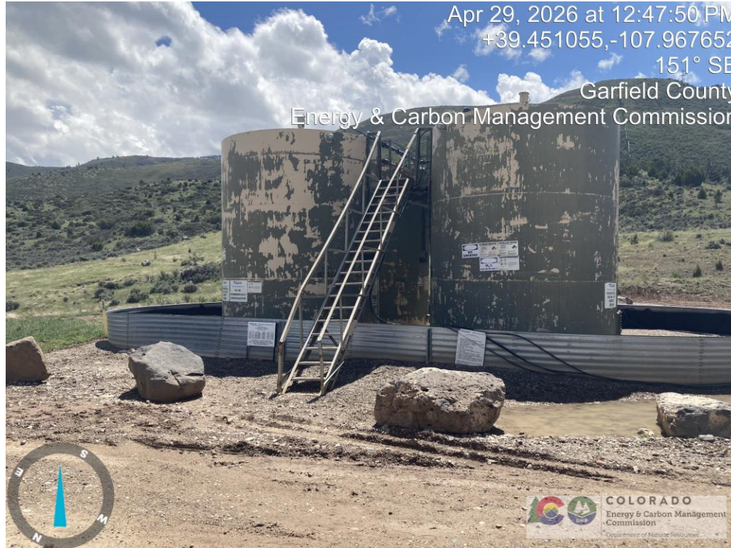
Paint deterioration and areas of rust.
