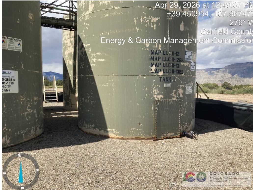
Paint deterioration and areas of rust.
