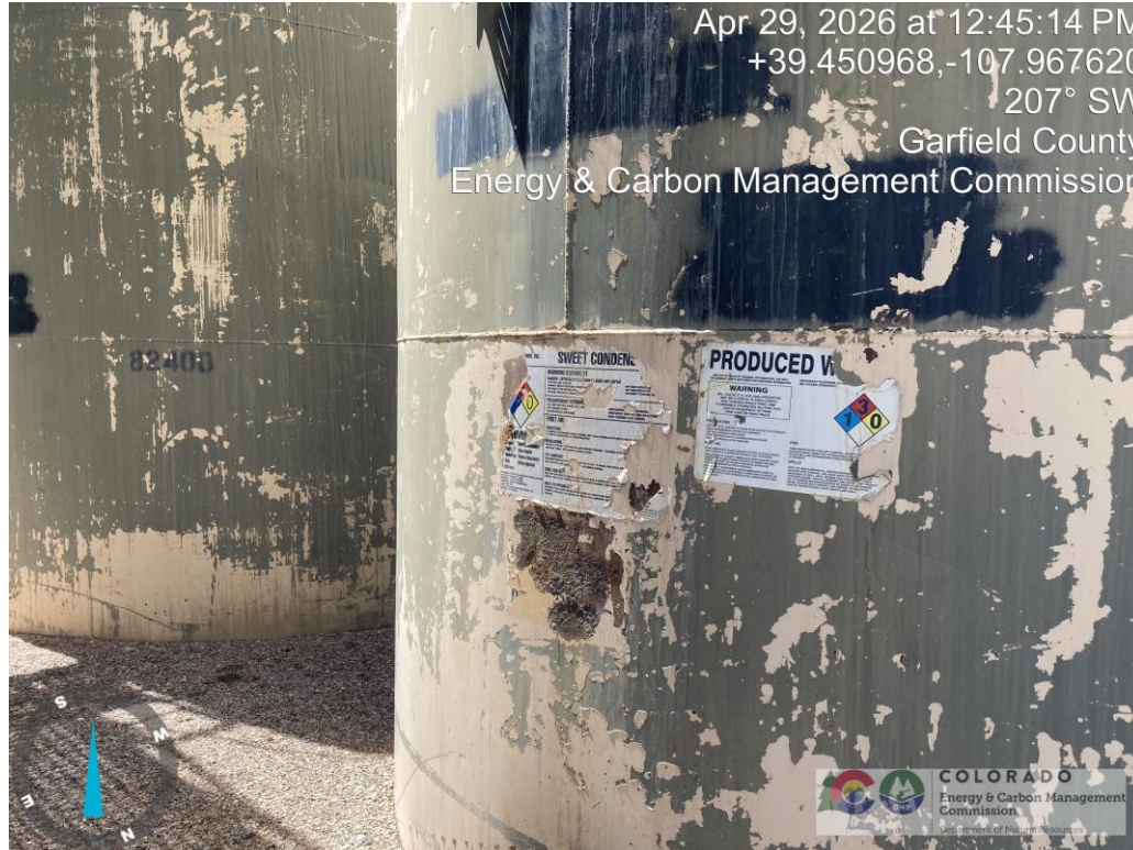
Paint deterioration and areas of rust. Torn and damaged labels.
