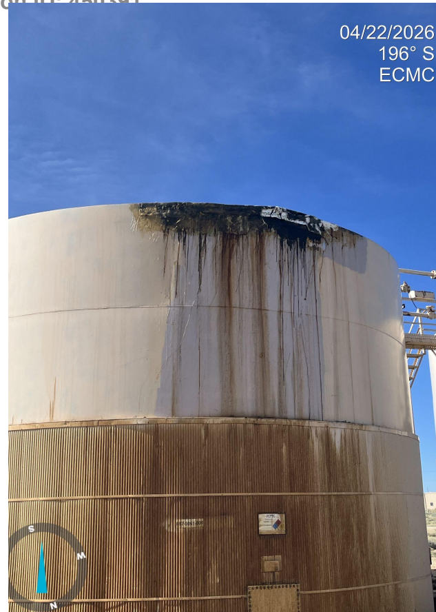
Photo 4. Photos 4-5 taken of the fiberglass patch on the tank.
