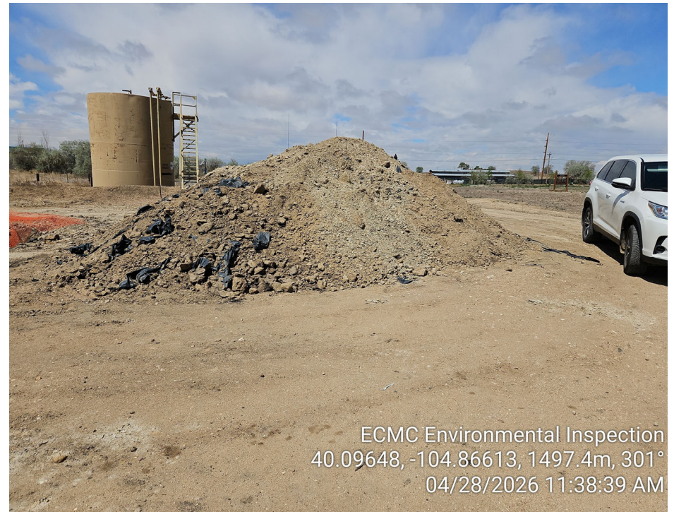
Photo 8 – Soil stockpile with no liner or stormwater BMPs.
