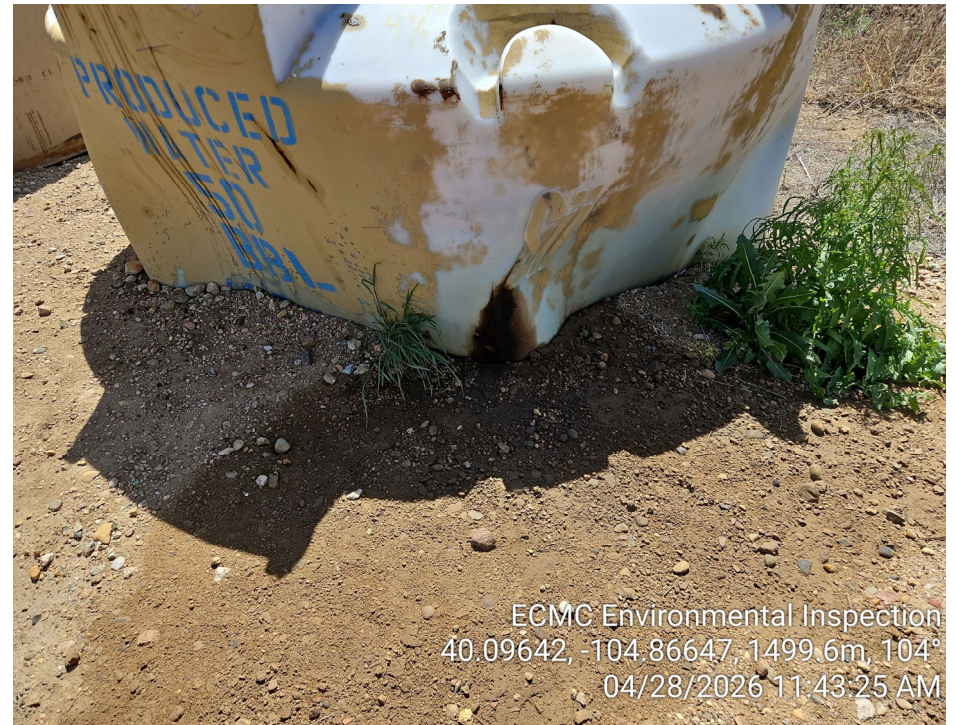
Photo 10 – Produced water tank is cracked. Stained soil next to tank. Weeds growing next to produced water tank.
