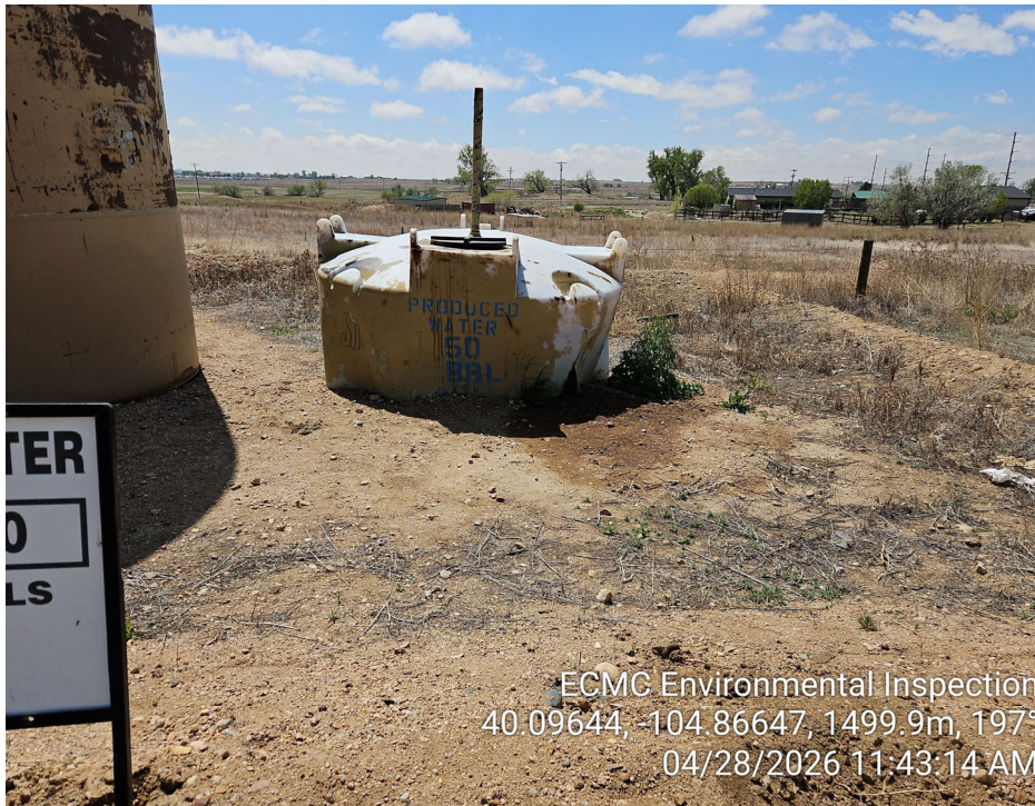
Photo 9 – Produced water tank is cracked. Stained soil next to tank.
