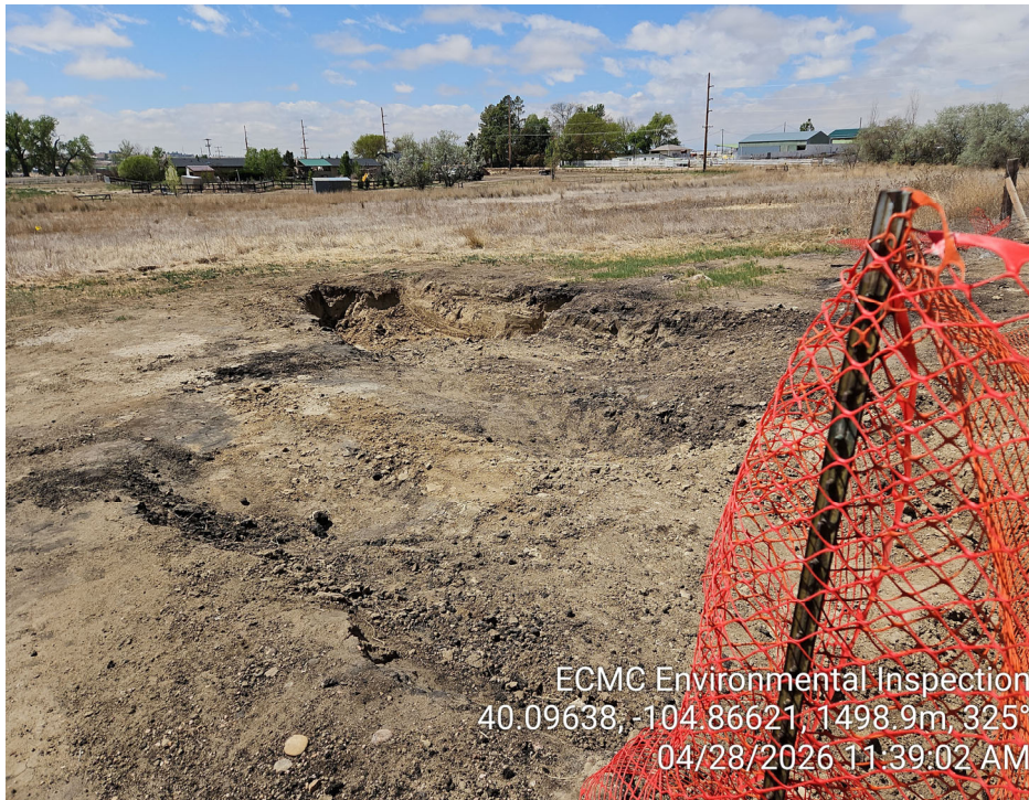
Photo 7 – Shallow excavation area with no fencing.
