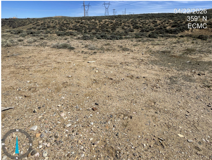
Photo 1. Photos 1-4 taken at the pad center, facing North, East, South and West illustrating the overview of the Location. The pad and access road have not been reclaimed; gravel remains.
