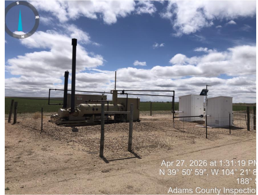
Photo #2 Separator & meter.
